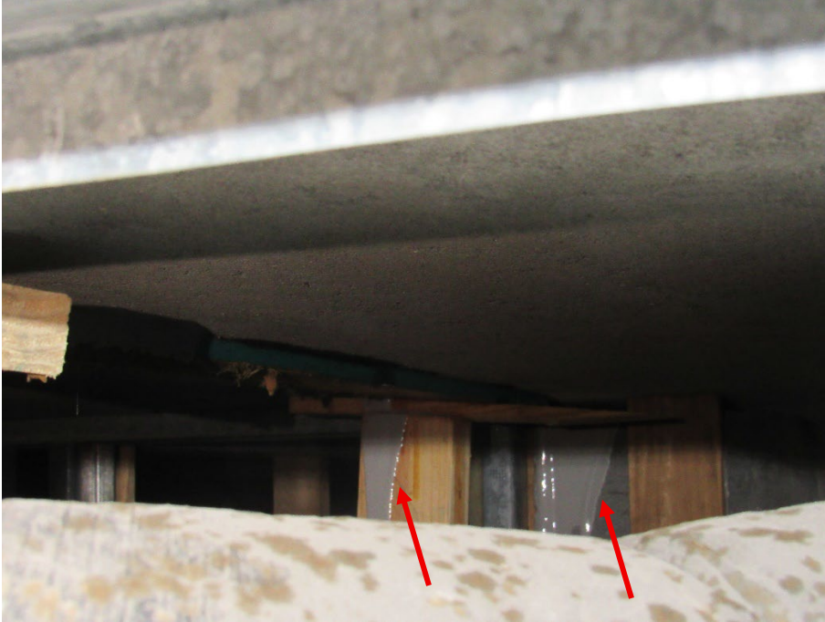
Observed epoxy leakage at formwork end point.
