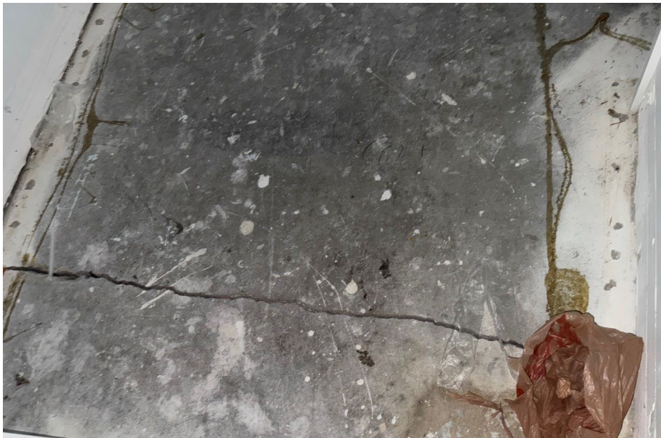
Observed interior structural slab crack.
