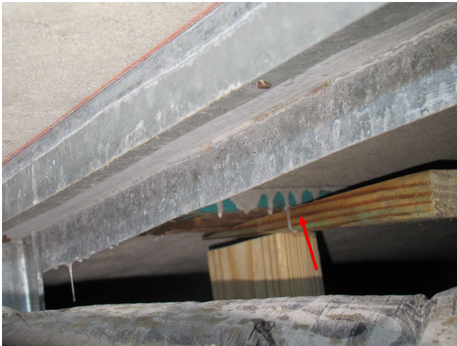
Observed epoxy leakage at unsealed formwork seams.
