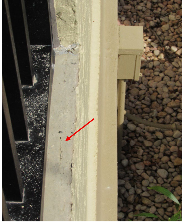
View of crack observed at the balcony slab edge.
