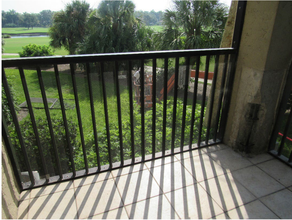
View of area of delaminated tiles.
