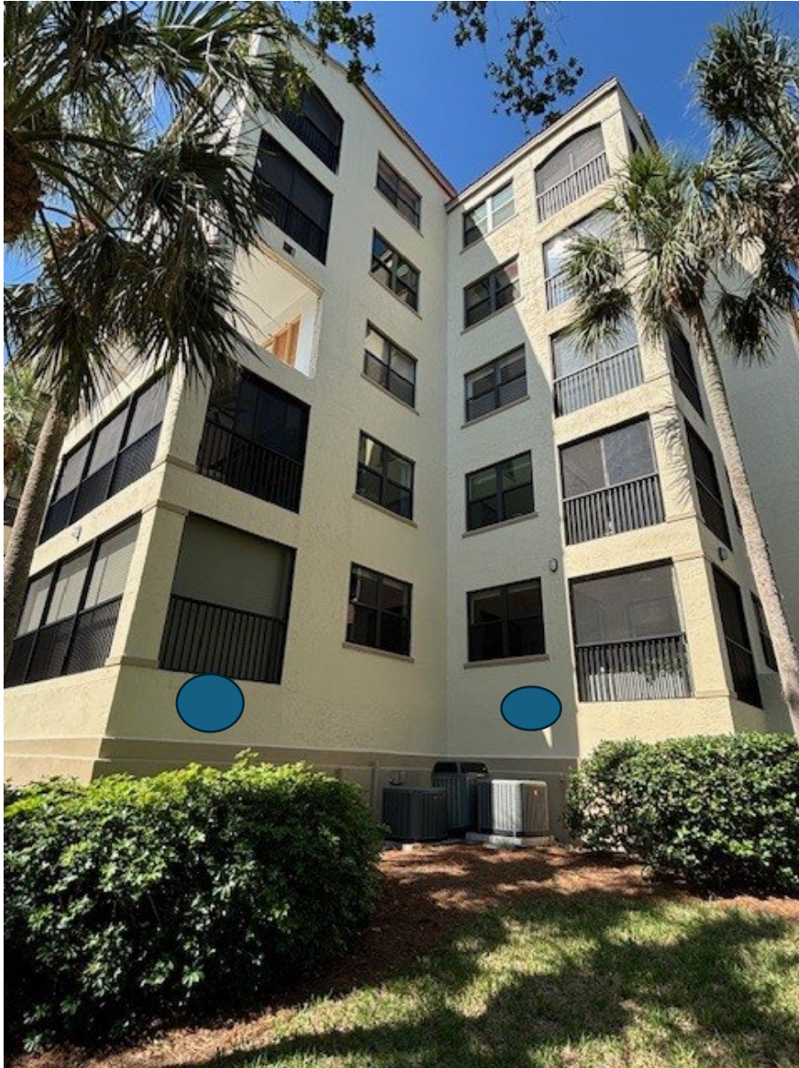
Picture 4, Locations where the stucco must be removed for further investigation.
