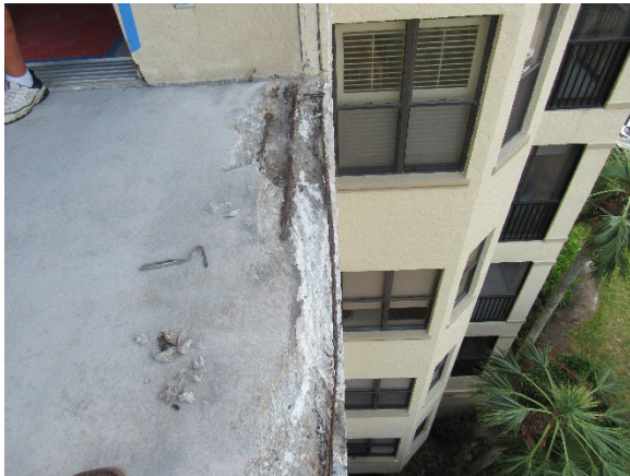
504 PT cables & corroded steel
