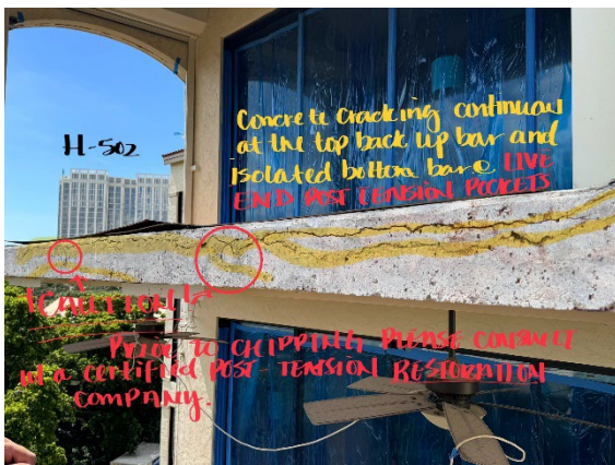
Extent of 502 damage
