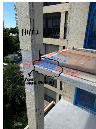
402 X-ray result w needed repairs
