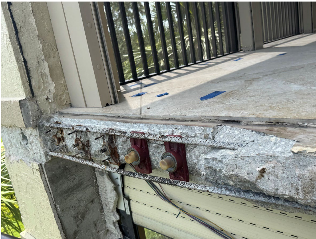
Unit F-305 – 7 identified PT cable anchors, 3 of which are cables extending through to Unit F-303. Remaining 3 severely corroded anchors observed to be replaced, suspected to end at wall of Unit F-303.
