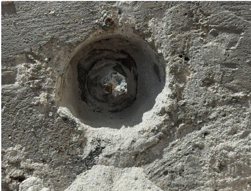
Unit F-304 – Initial observations of the band-line cable pockets show signs of corrosion on the anchors at the cable pockets.
