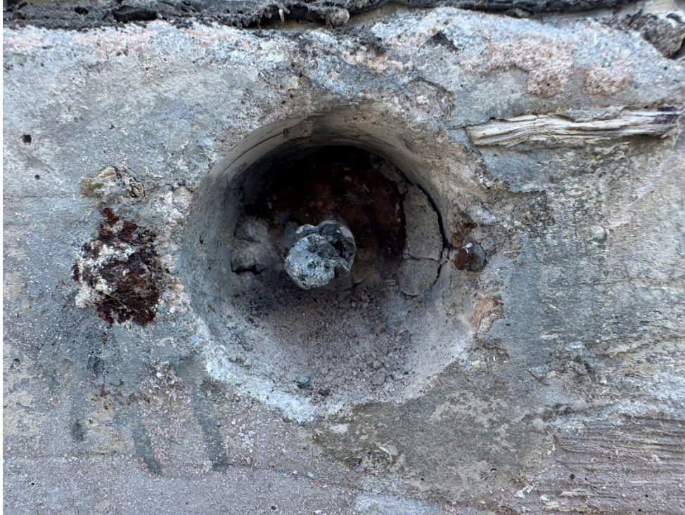
Unit H-501 – Observed severely corroded cable anchor
