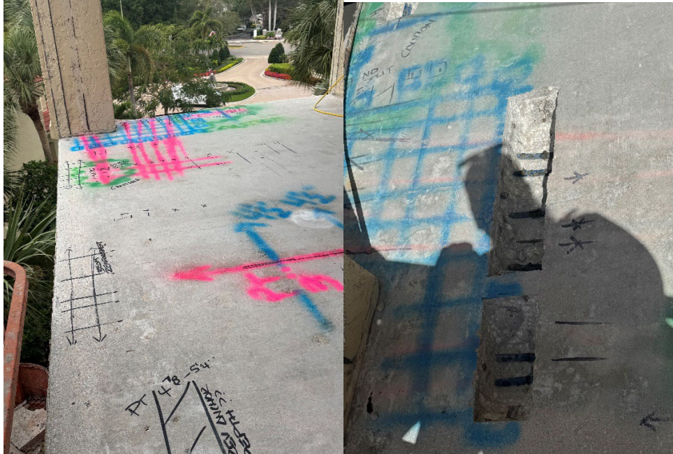
Unit F-301 – Concentration and clustering of reinforcement bars and PT cables identified through GPR scanning in the south corner of balcony
