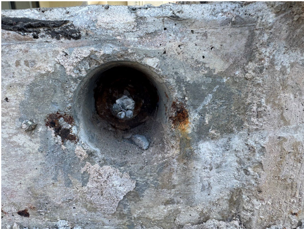
Unit H-501 – Observed severely corroded cable anchor
