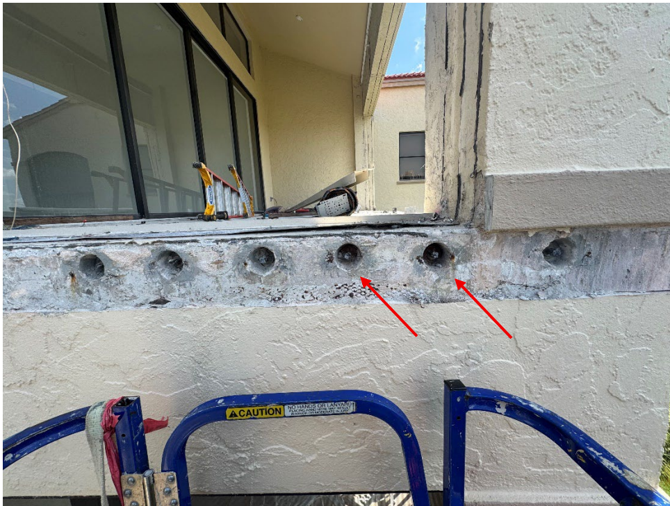
Unit H-501 – Southwest slab edge, exposed cable anchor pockets
