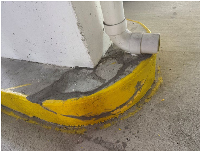
Building F – Ground Level Garage: Structural distress observed
