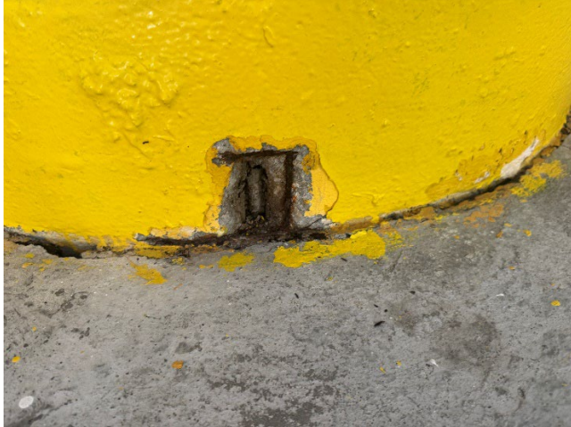
Building H – Ground Level Garage: Structural distress observed
