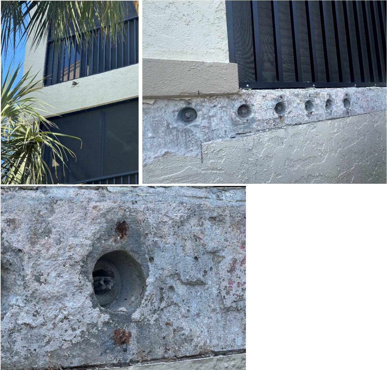
Unit F-305 condition: damage observed at balcony slab edge. Cable observed with wedges released.
