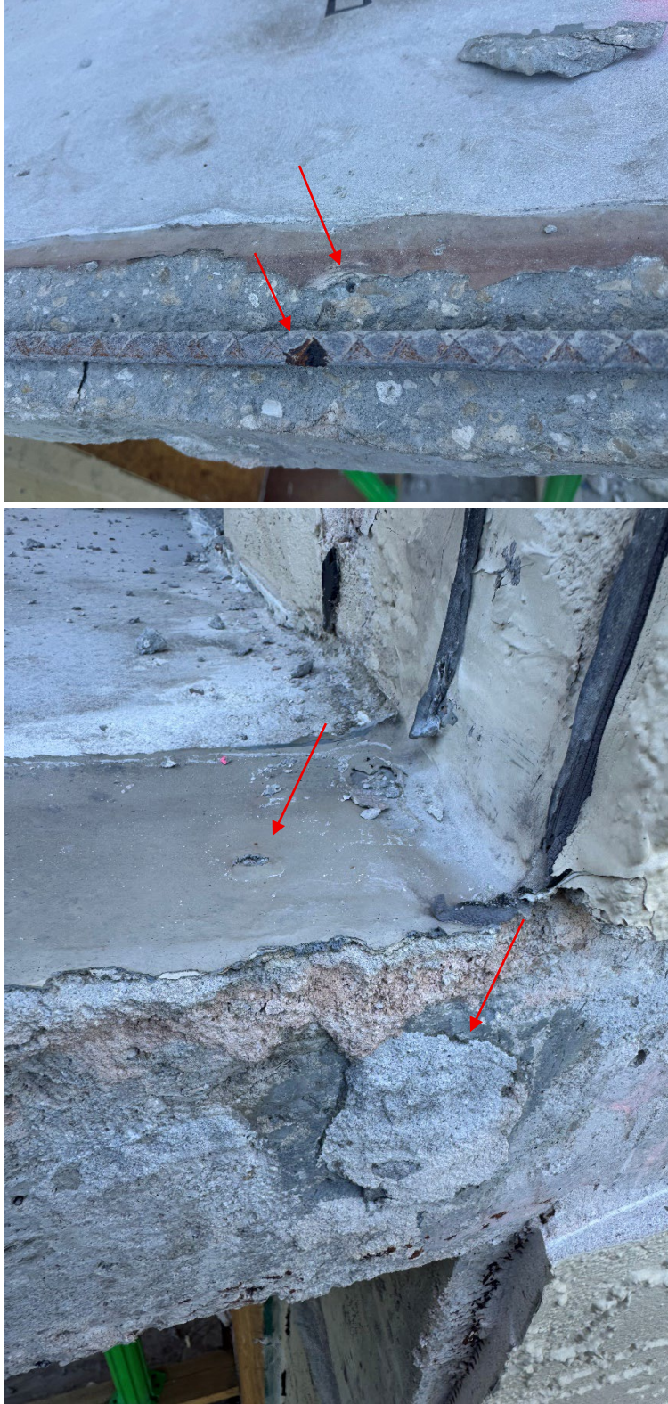
Unit F-303 balcony slab edge: corrosion patterns and PT pockets aligned with the locations of fastener holes.
