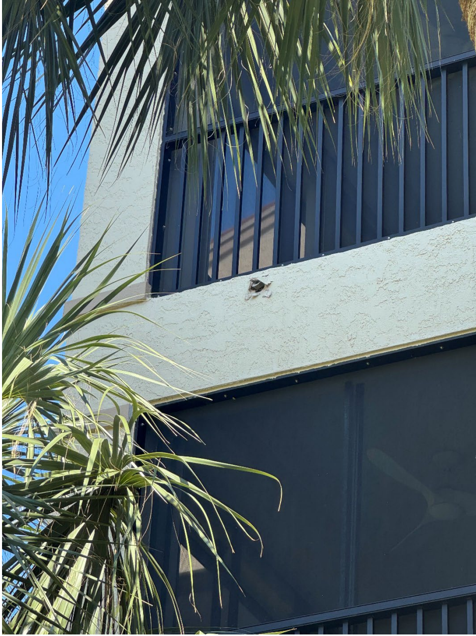
Unit F-305 condition: damage observed at balcony slab edge. Full exposure will be necessary for proper assessment.
