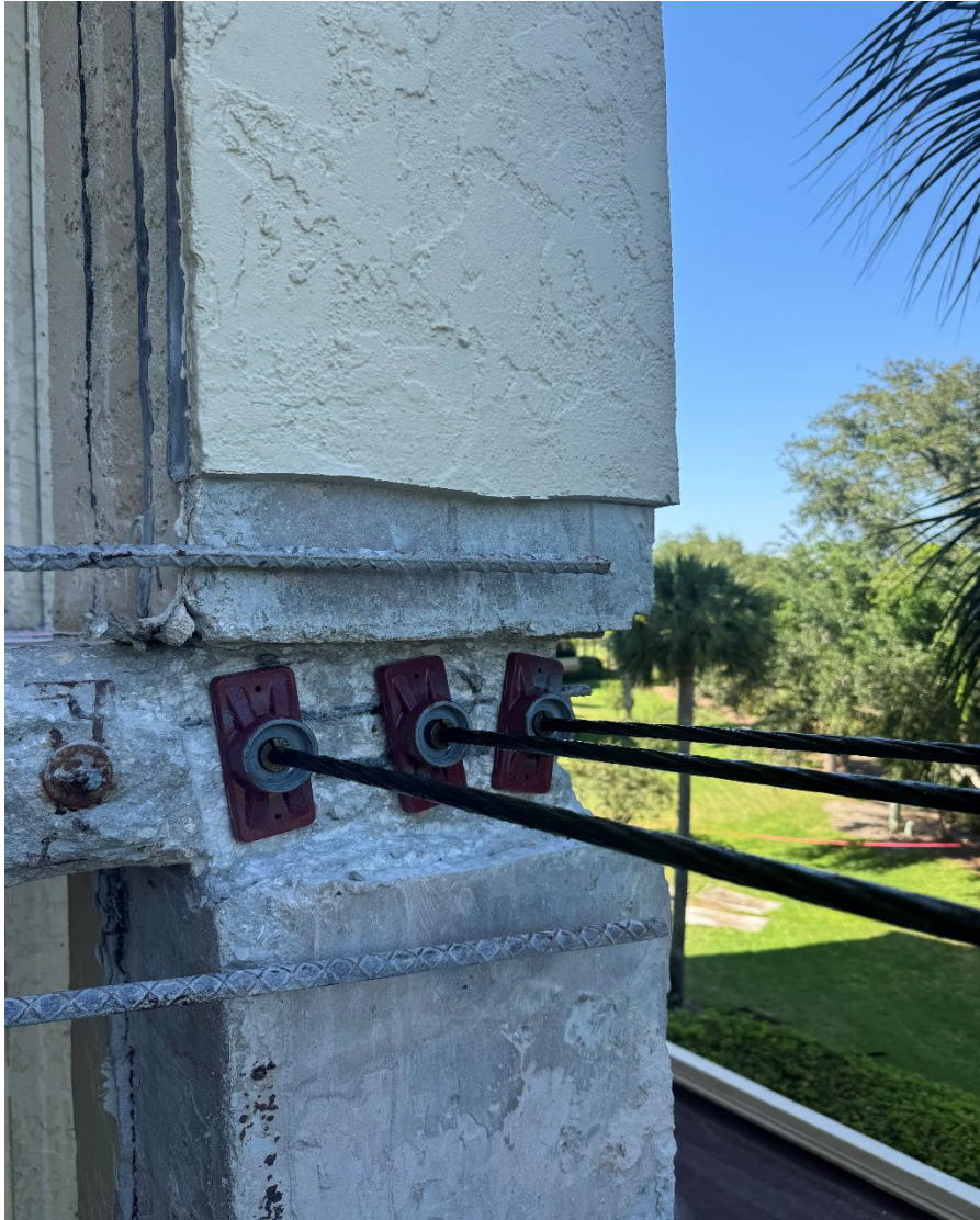
Unit F-303 balcony slab edge: 3 original uniform cables emanating from the column.
