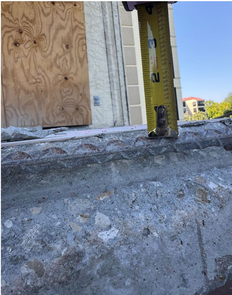
Unit F-303 balcony slab edge: Insufficient coverage on slab edge reinforcement not achieving the required 2 inches.
