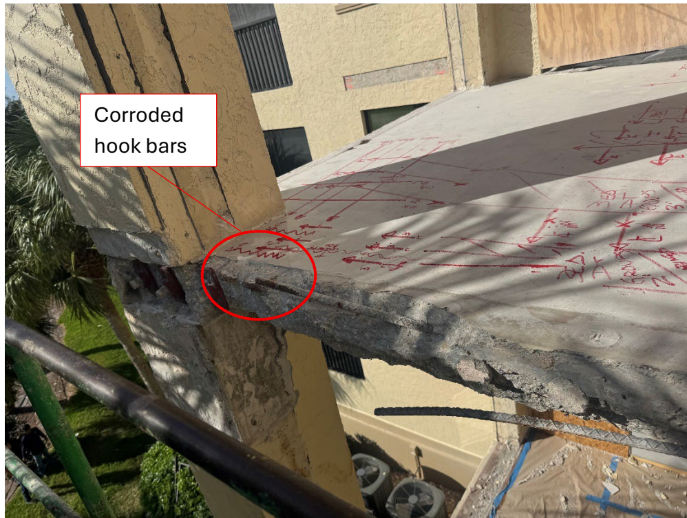
Slab edge conditions at Unit F-303 balcony showing corroded hook reinforcement bars and area of potential delaminated concrete.
