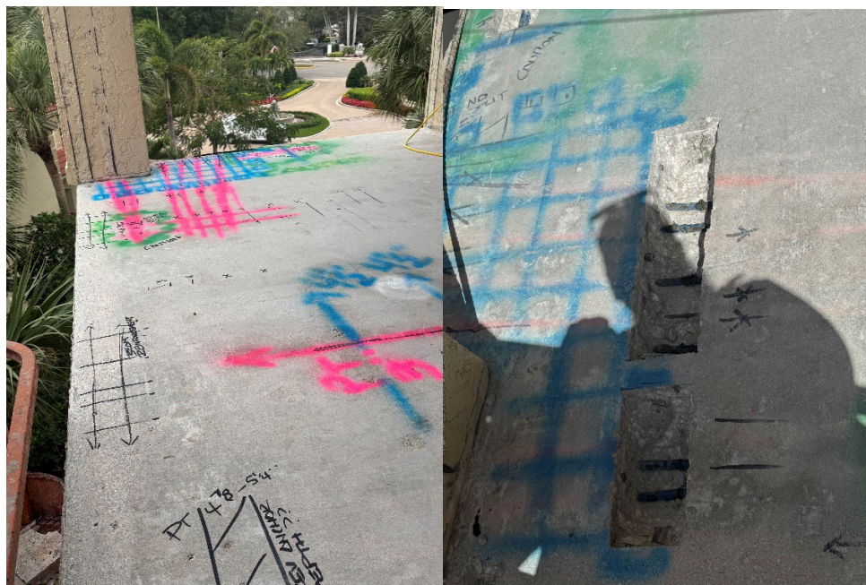
Concentration and clustering of reinforcement bars and PT cables identified through GPR scanning in the south corner of balcony, Unit F-301.
