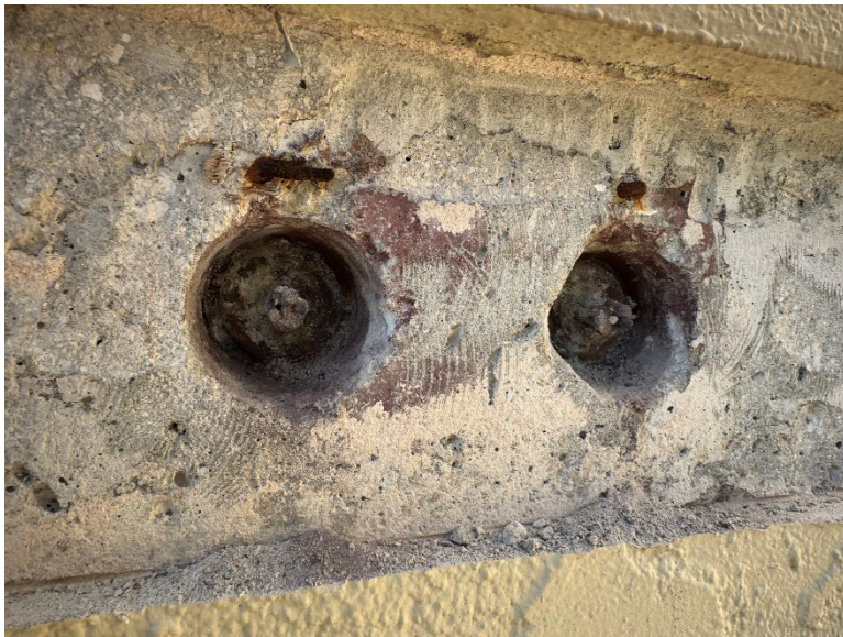
Unit F202: Observed deterioration/corrosion of the post tension cable anchor pockets.
