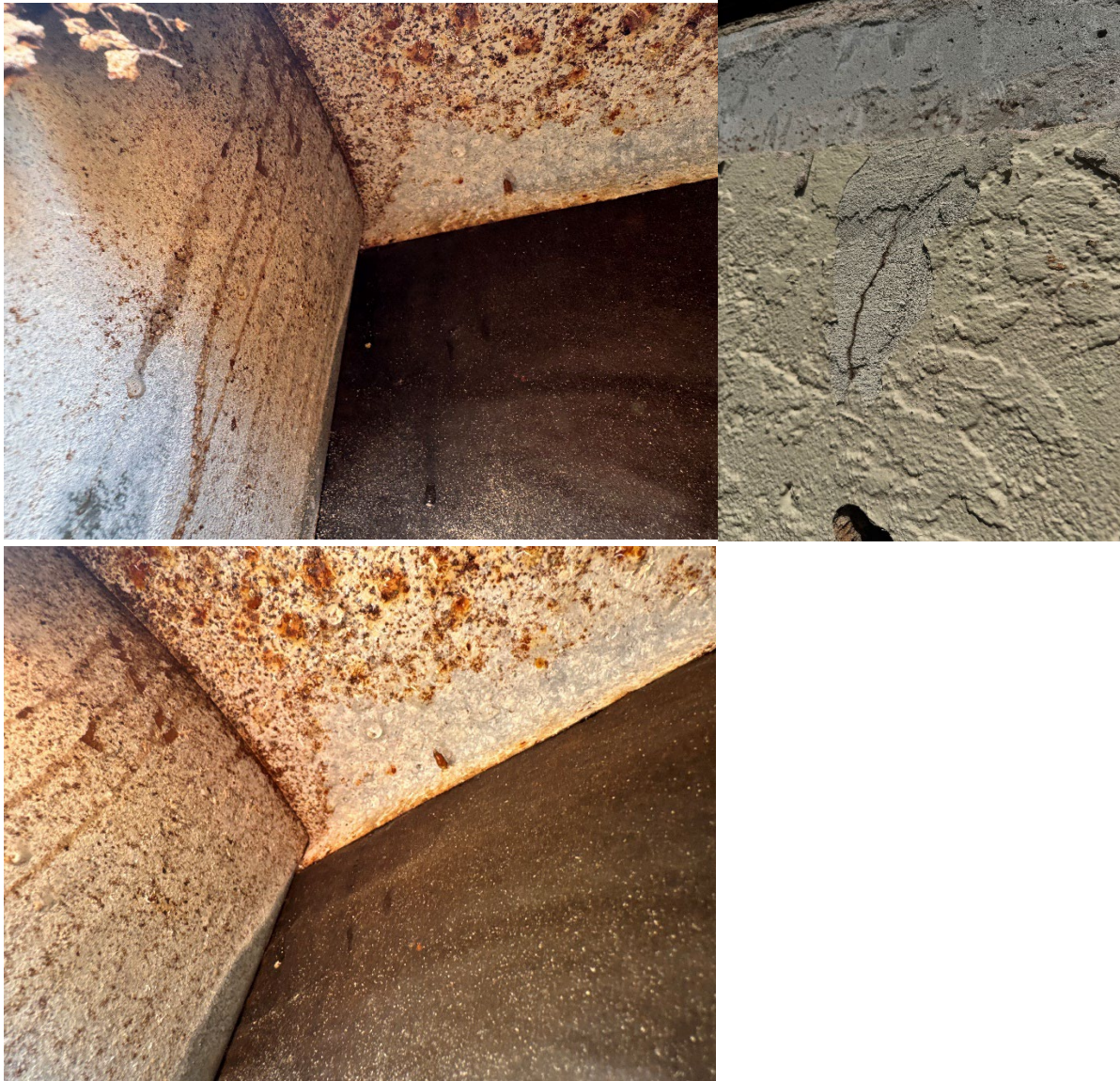
Unit F102: Observed corrosion of the metal framing and structural distress.
