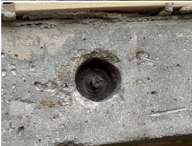
Fourth Floor Walkway: Observed deterioration/corrosion of the post tension cable anchor pocket.
