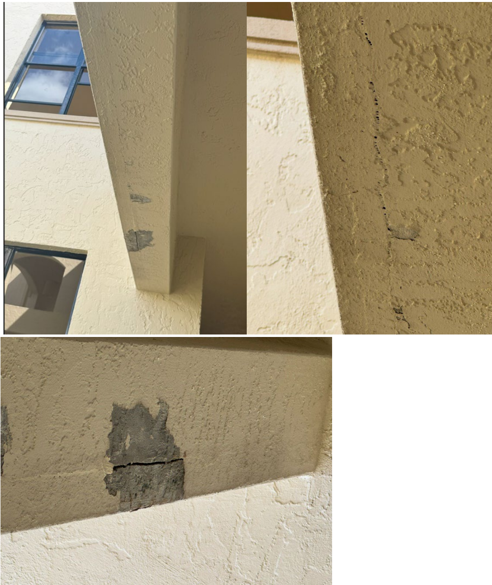
Fourth Floor Walkway: Previously observed delamination and linear crack along header.
