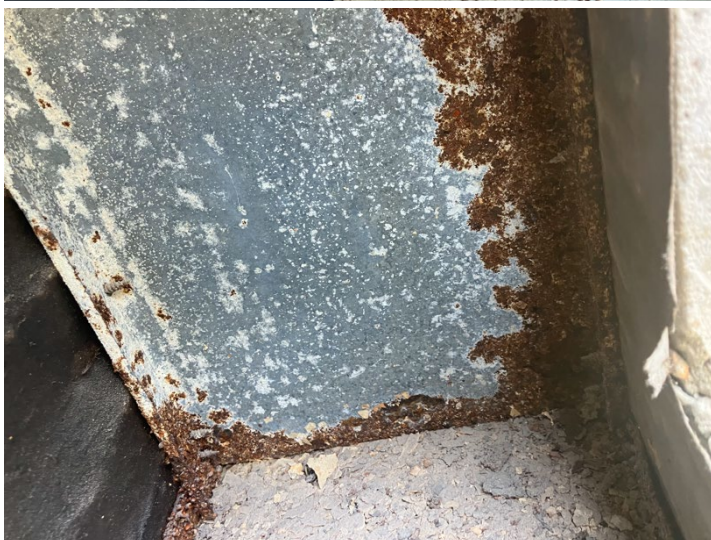
Right Header – Signs of severe corrosion of the metal framing.
