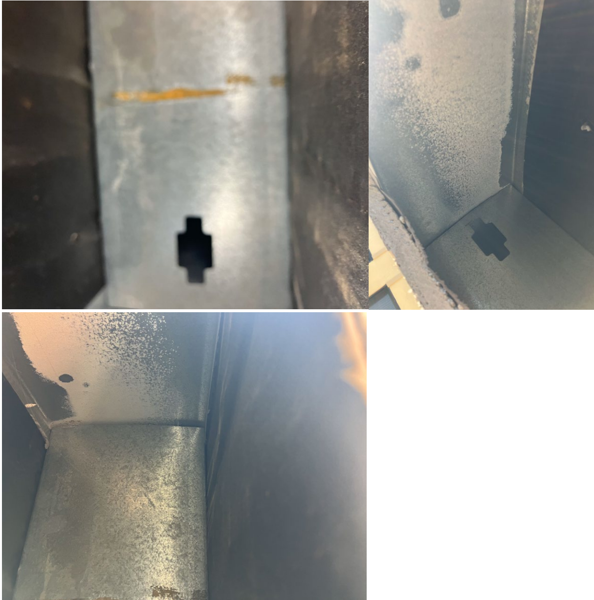
Left Header – No signs of corrosion and deemed in good condition.
