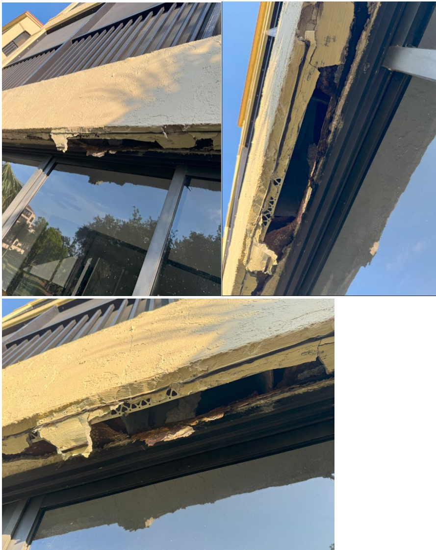
Larger Header – Signs of severe corrosion and deterioration of metal framing.
