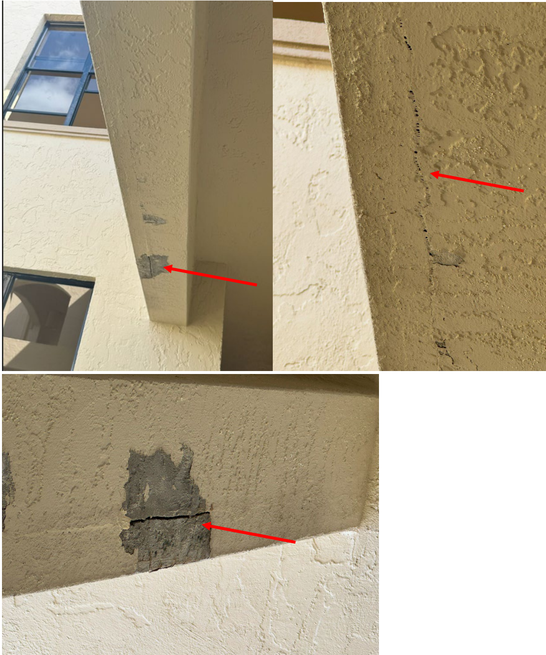
Fourth Floor Walkway: Observed delamination and linear crack along header.
