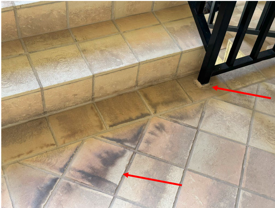
Area Under Staircase: Signs of water ponding and possible water intrusion.
