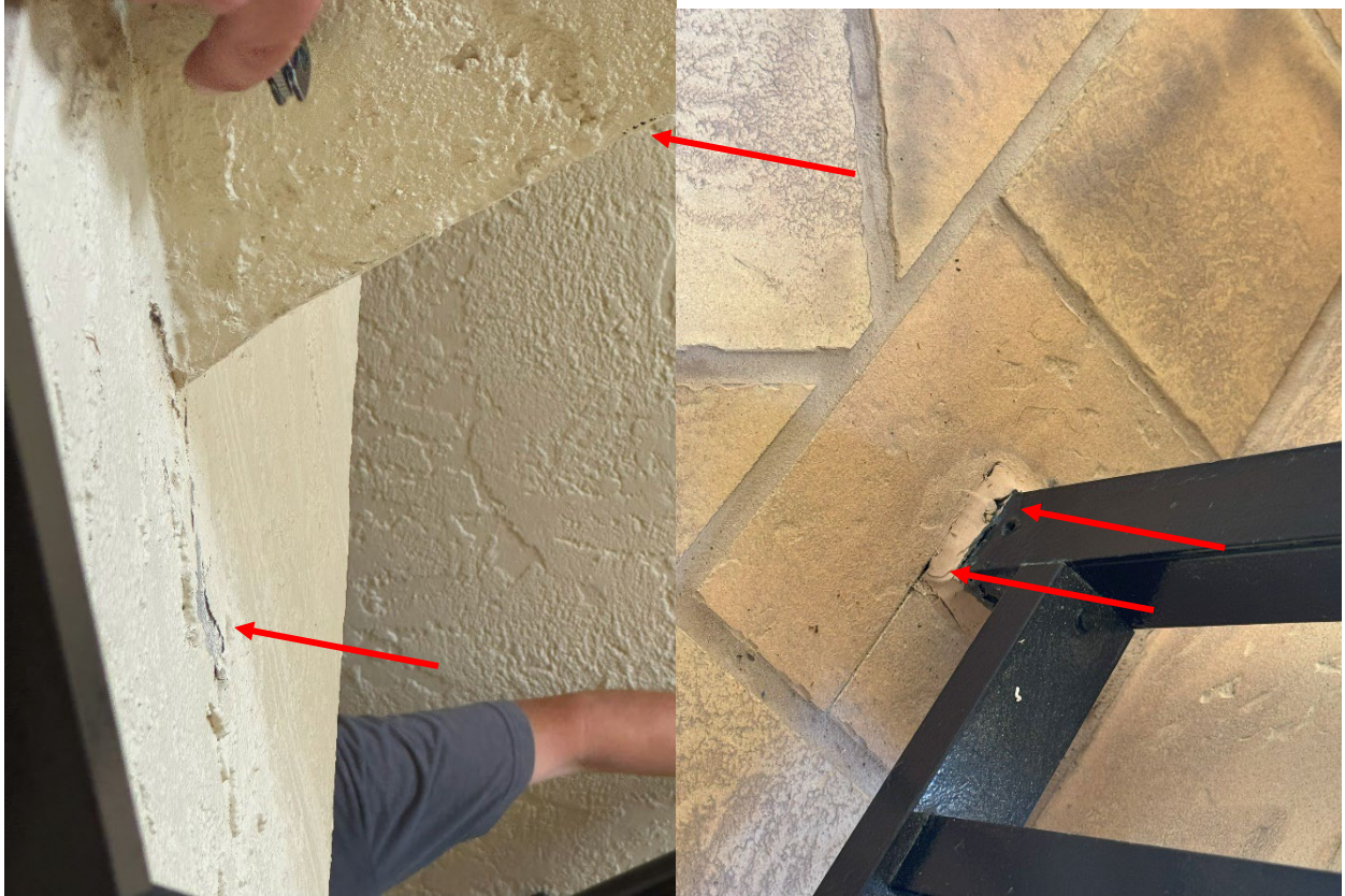
Area Under Staircase: Observed stucco delamination and possible water intrusion at railing post.
