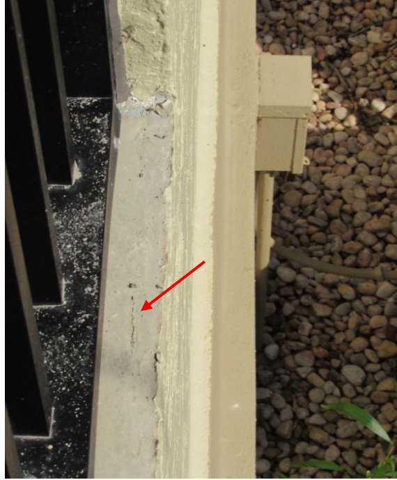
View of initial signs of distress at balcony deck edge – minor cracks.
