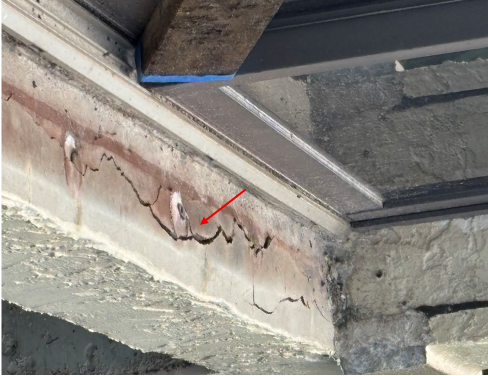
View of structural distress observed at balcony deck edge along fastener points.
