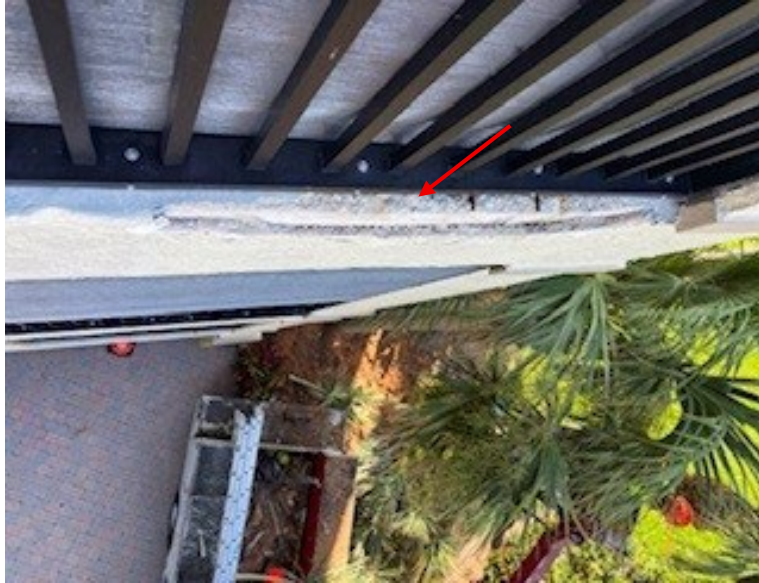
View of exposed balcony deck edge steel reinforcement bar and concrete spall.
