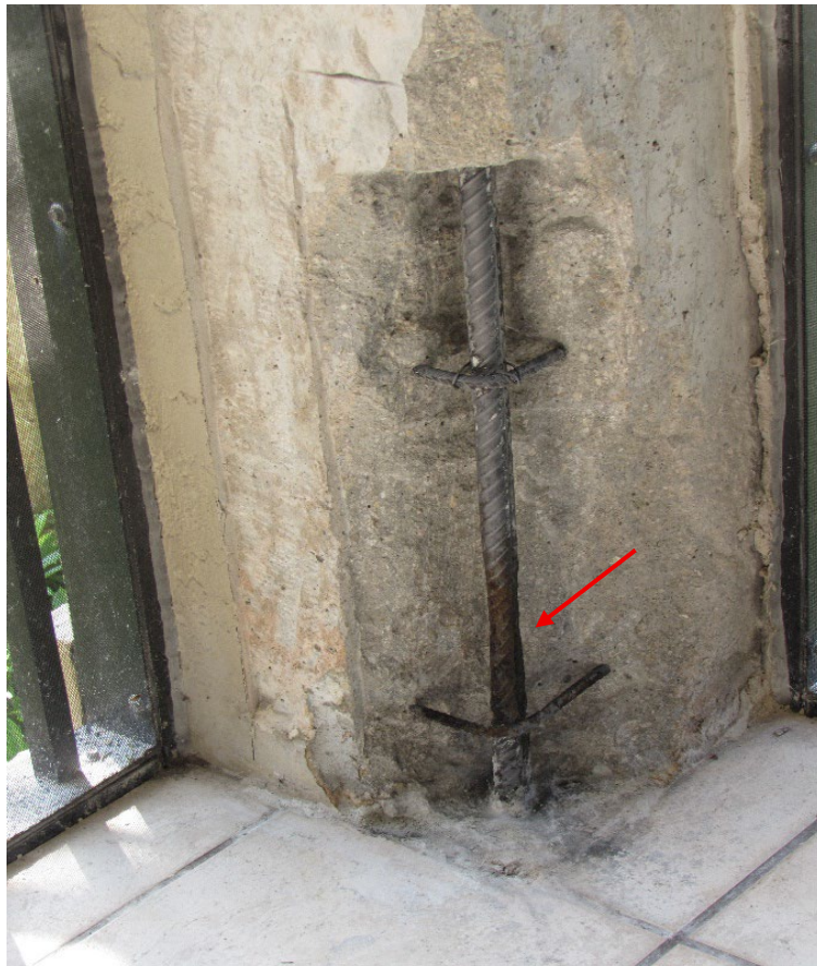
View of corroded steel reinforcement bar and distressed concrete at balcony column.
