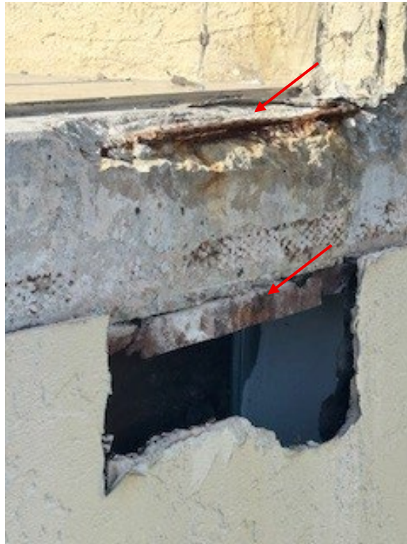
View of corroded steel reinforcement bar, deteriorated concrete, and header framing.
