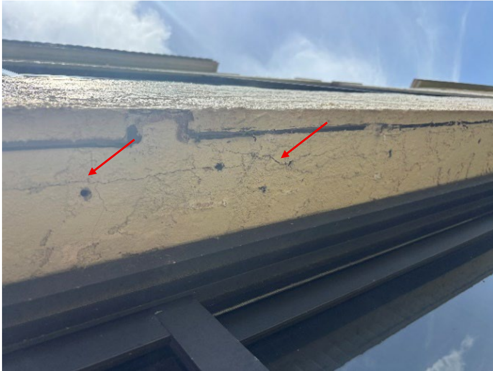
View of initial signs of distress on headers - stucco cracks along the fastener points.
