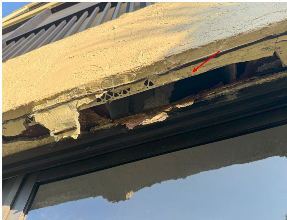
View of deterioration of header observed after further investigation.
