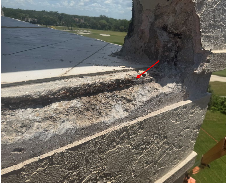
View of corroded steel reinforcement bar along balcony deck edge.
