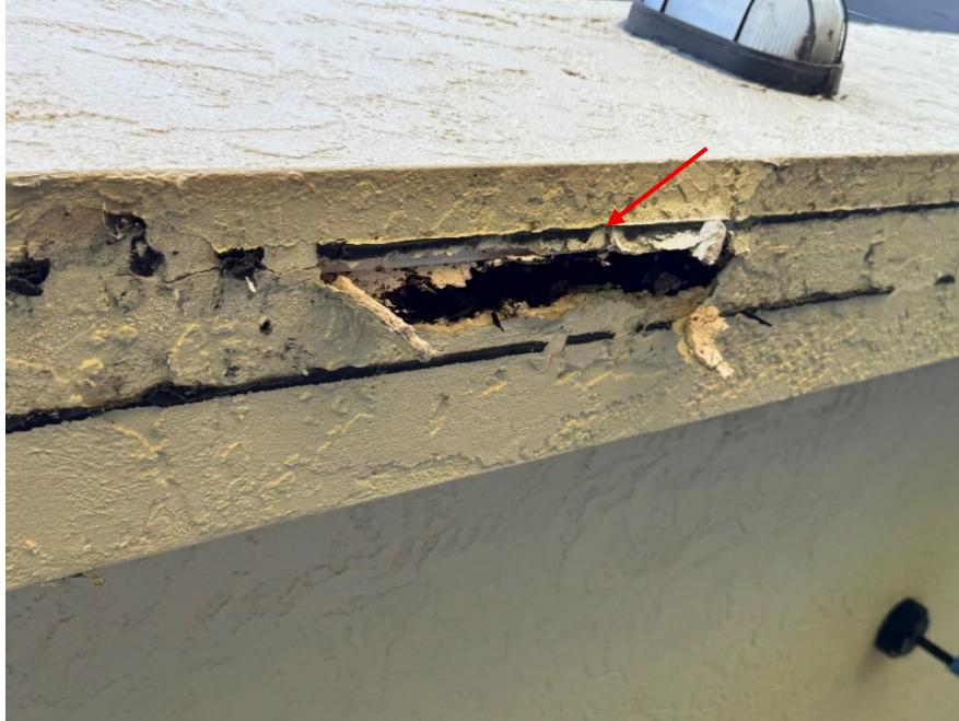
View of deterioration of header observed after further investigation.
