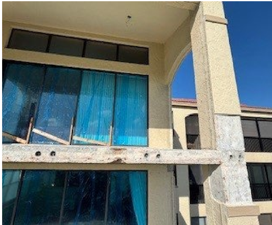
Typical view of compromised post-tension cables along balcony deck edge.
