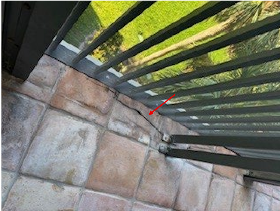
View of cracked/delaminated tiles stemming from shutter system fastener points.
