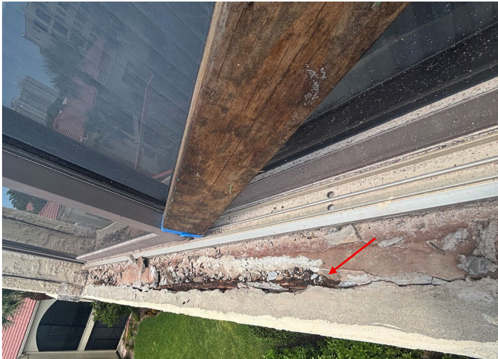
View of structural distress parallel to corroded steel reinforcement bar.
