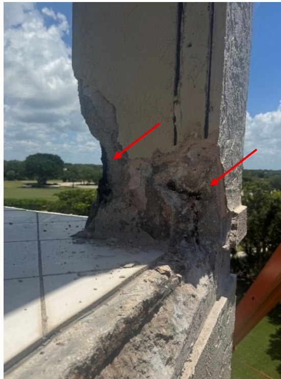
View of corroded steel reinforcement bar and distressed concrete at balcony column.
