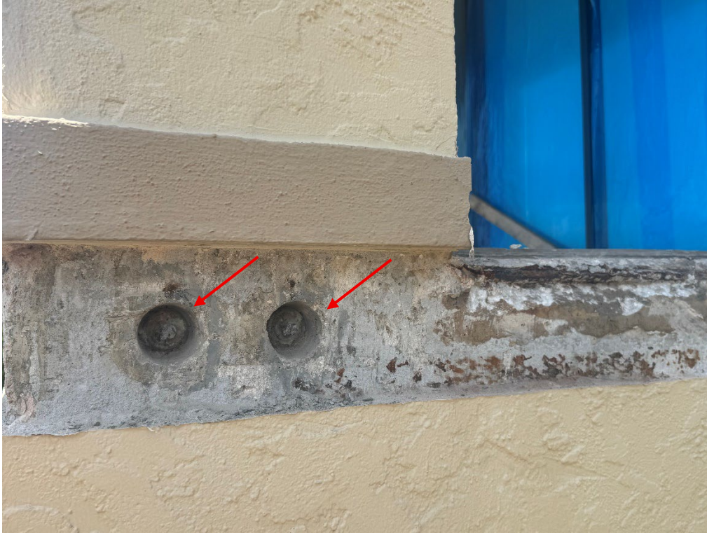
View of post-tension cable pockets with deteriorated cement and signs of corrosion.
