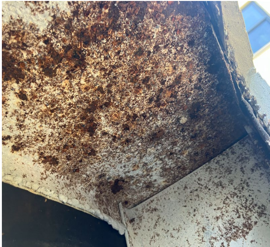
View of condition of header metal framing observed.
