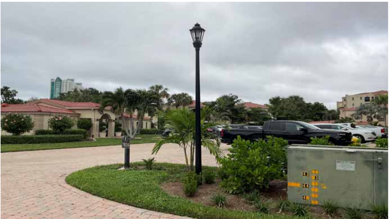
Light Pole & Fixture - Parking Lot
