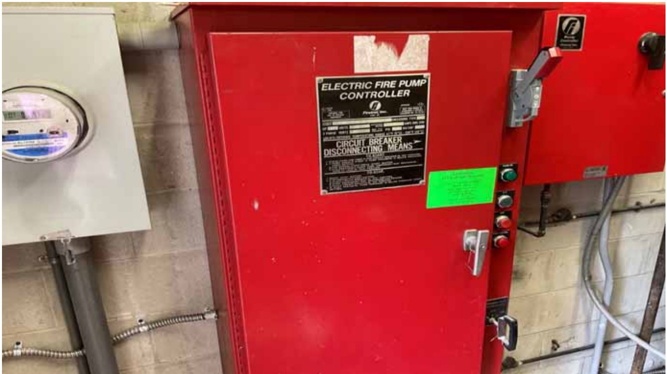
Building F Fire Pump Controller
