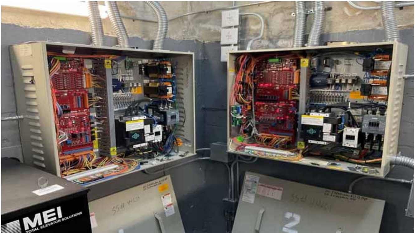
Building F Elevator Equipment
