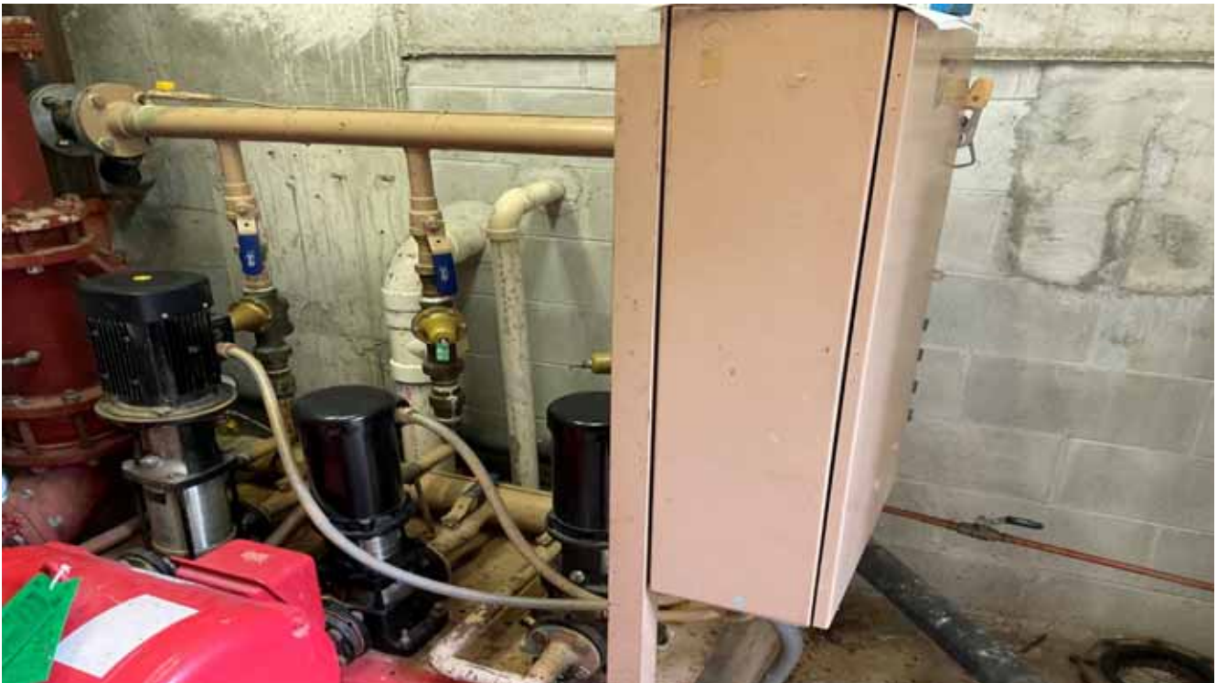
Building F Domestic Water Pump System
