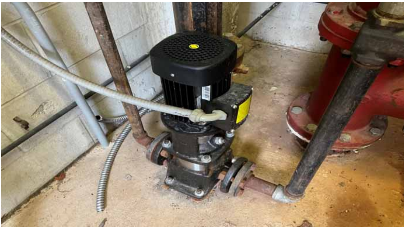
Building F Fire Jockey Pump
