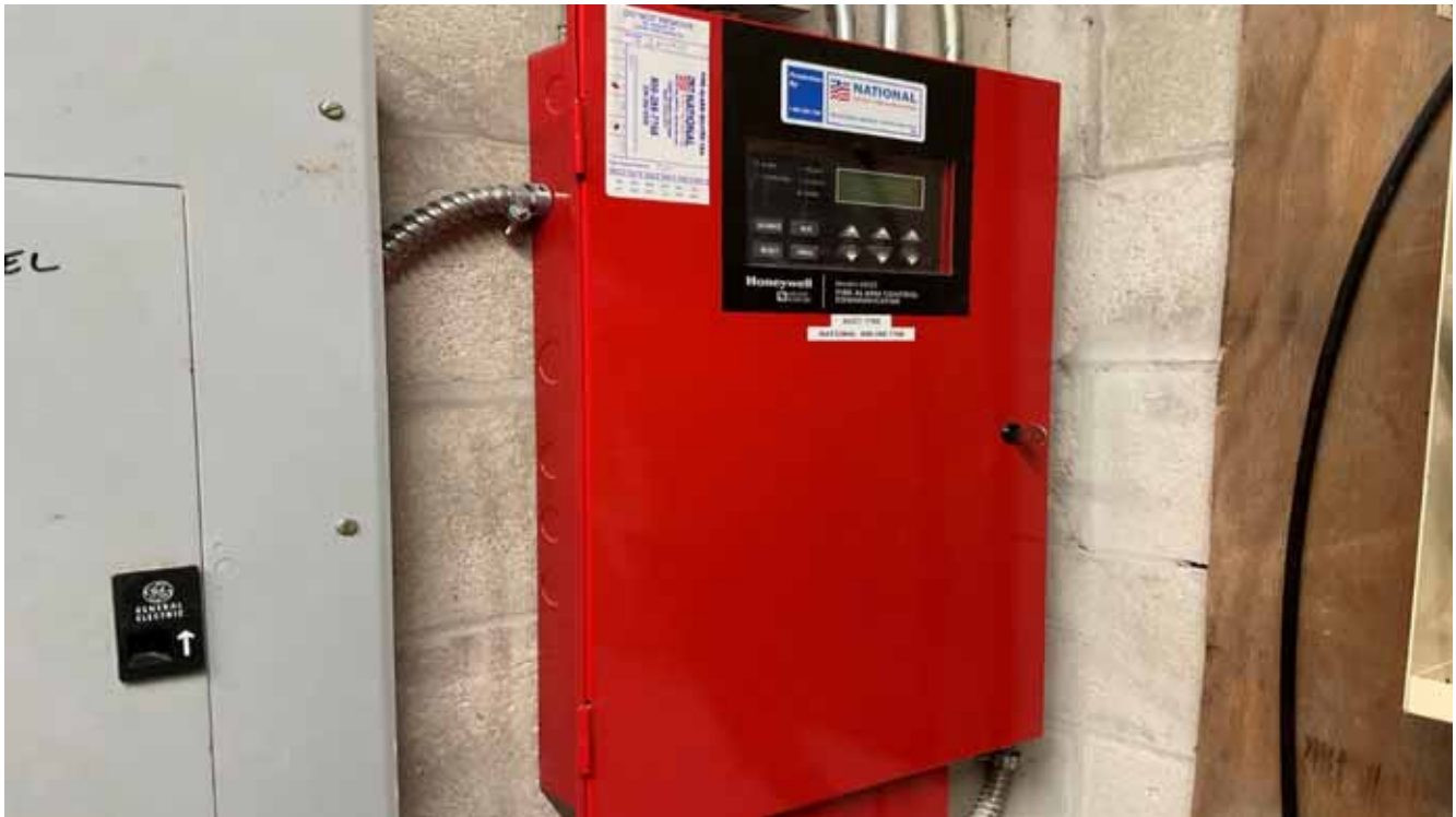
Building C Fire Alarm Panel
