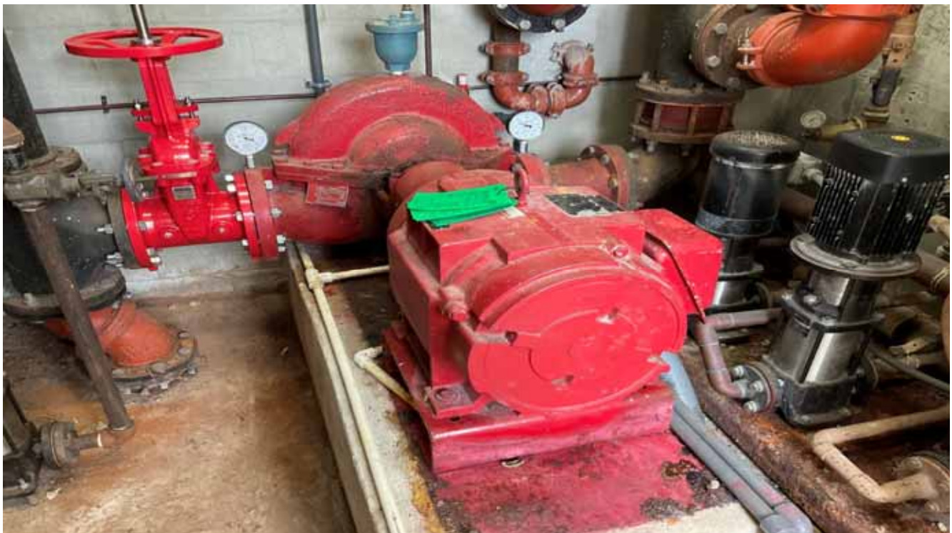
Building D Fire Pump
