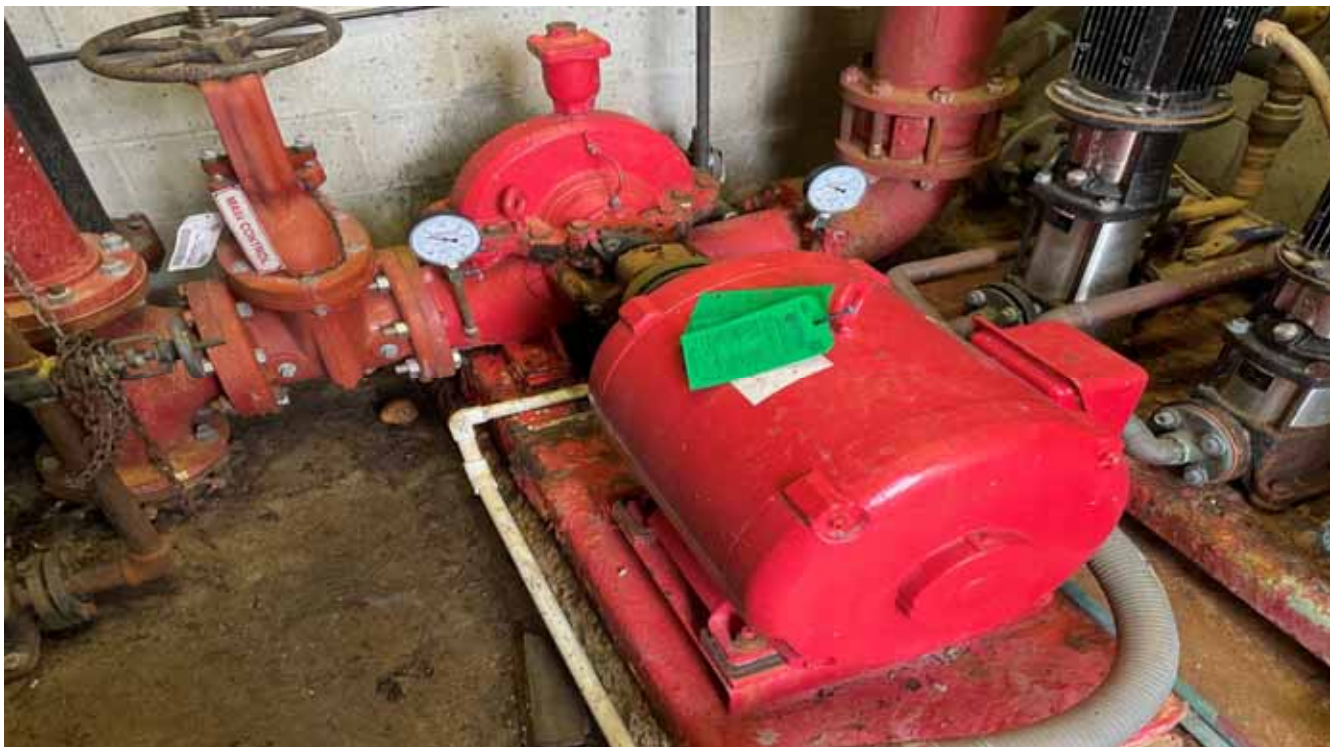
Building H Fire Pump
