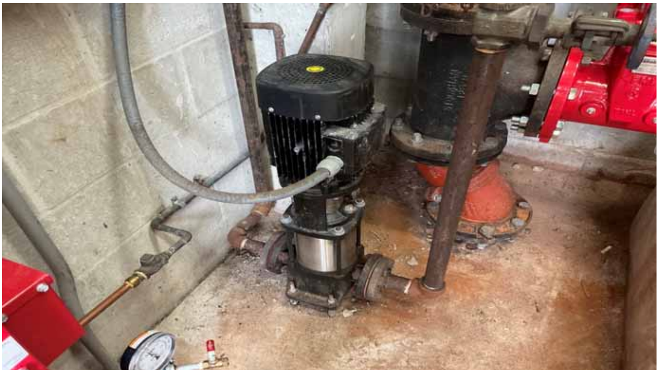
Building D Fire Jockey Pump
