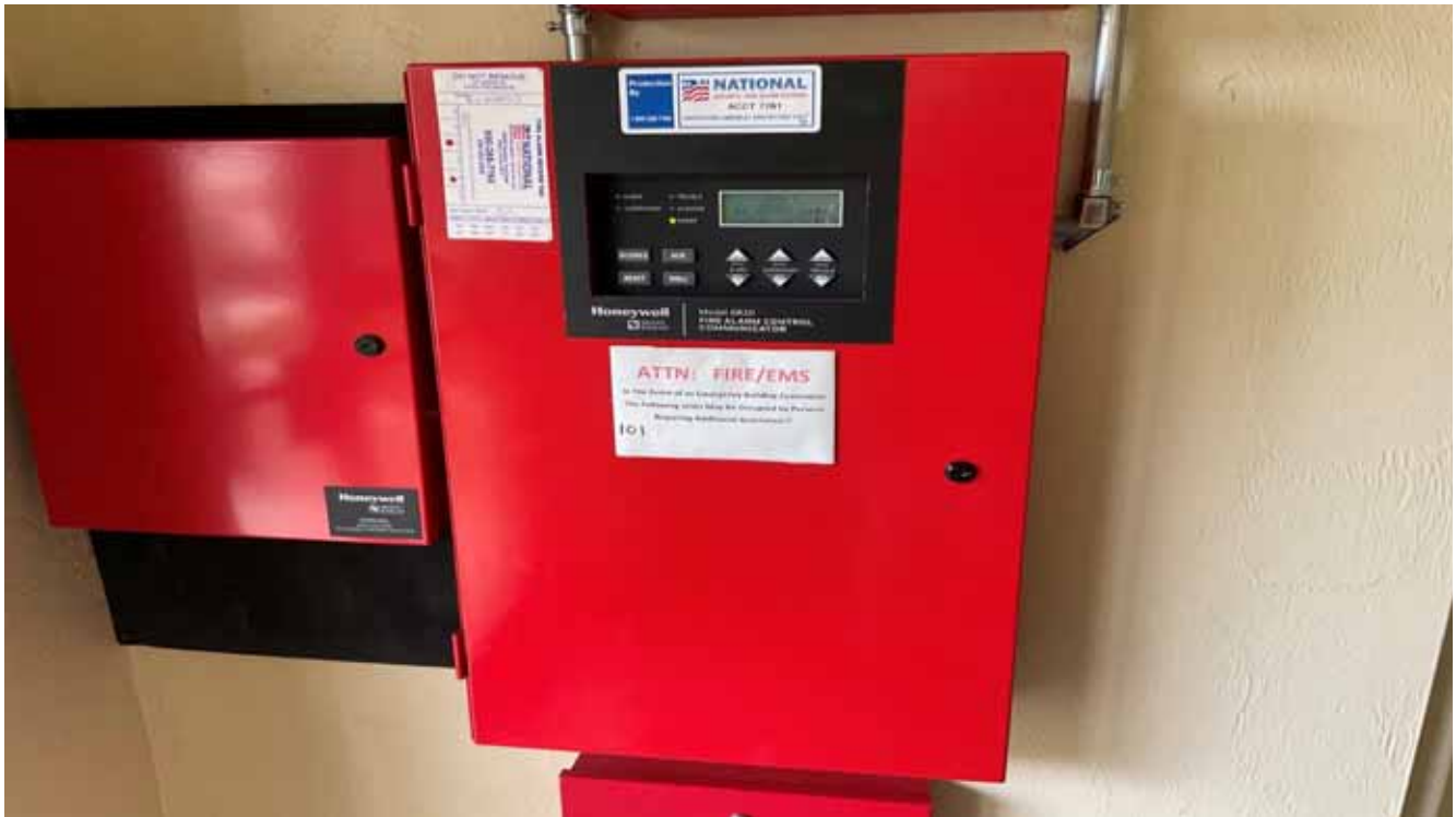
Building H Fire Alarm Panel
