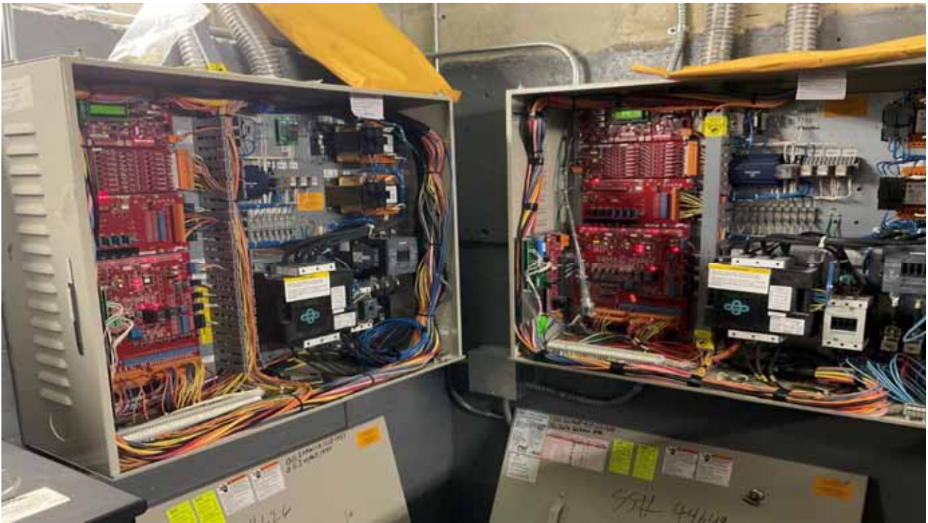
Building D Elevator Equipment
