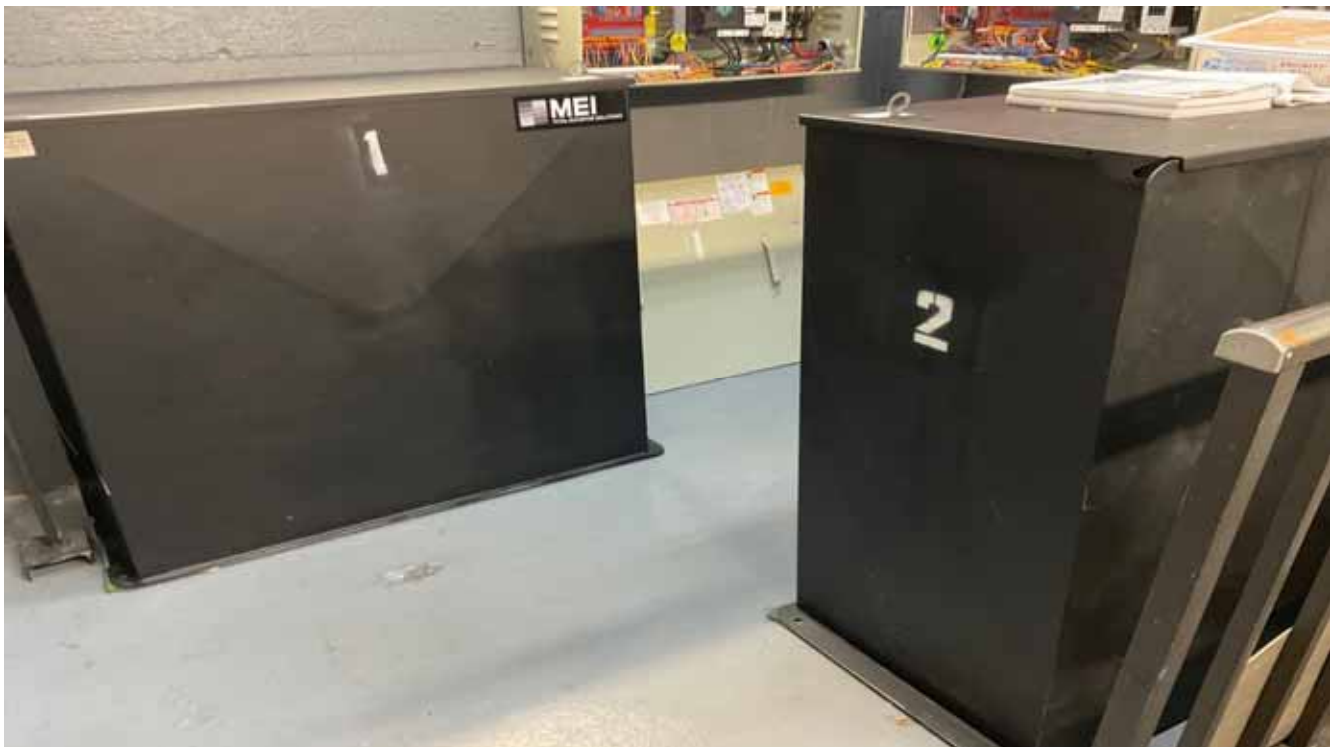
Building H Elevator Equipment
