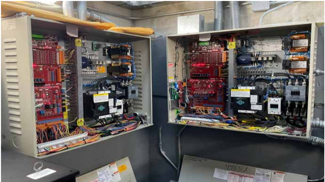
Building H Elevator Equipment
