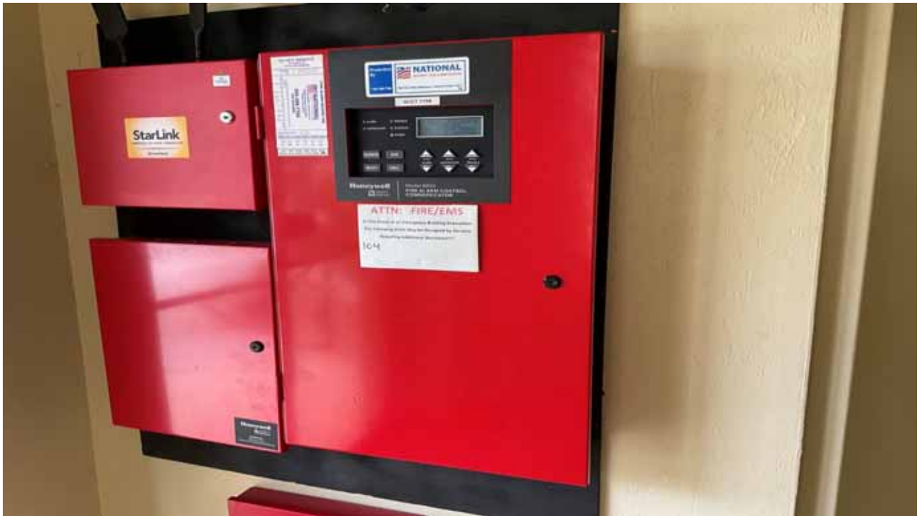
Building D Fire Alarm Panel
