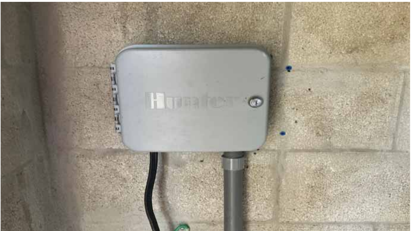
Irrigation Control Station (1 of 6)
