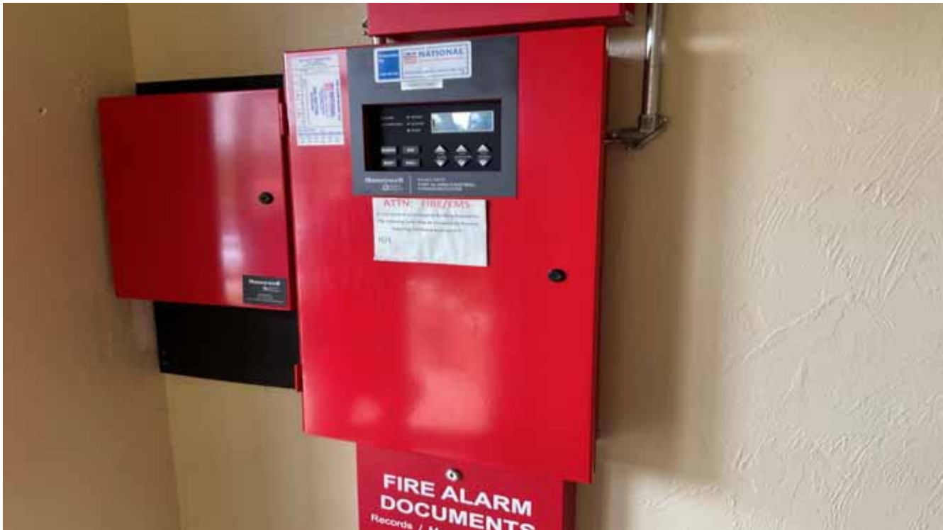
Building F Fire Alarm Panel
