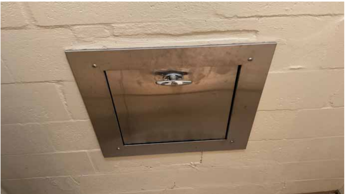
Building D Trash Chute Door
