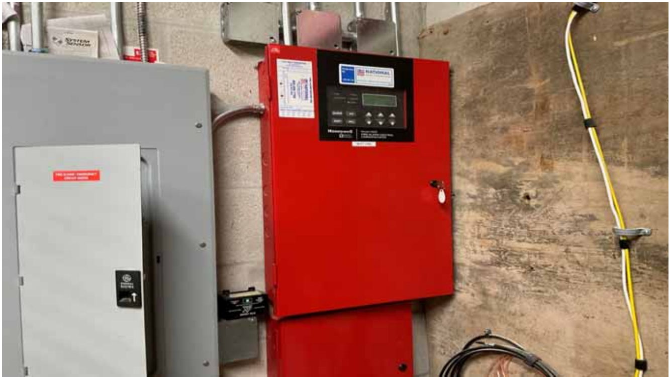
Building E Fire Alarm Panel
