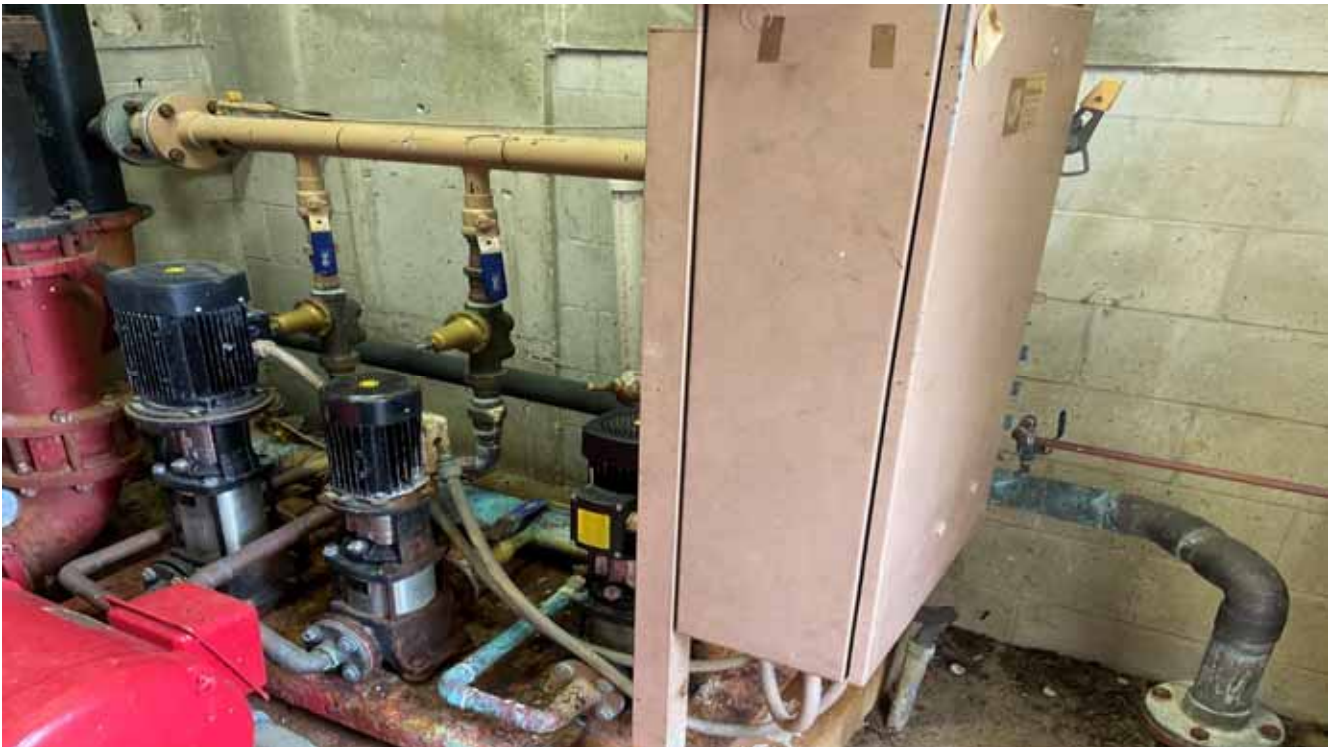
Building H Domestic Water Pump System
