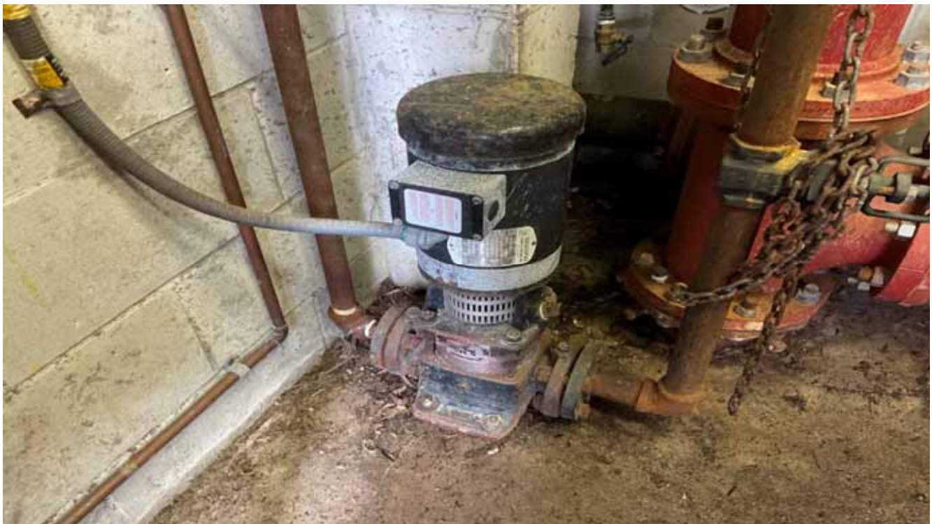
Building H Fire Jockey Pump
