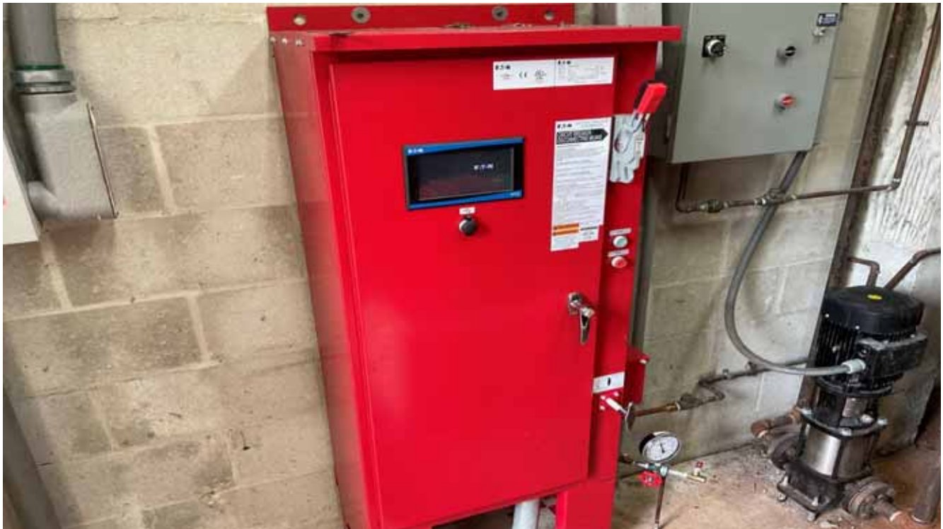
Building D Fire Pump Controller
