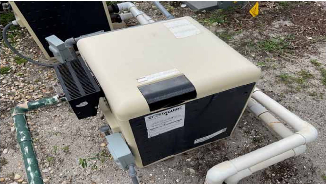
Spa Equipment, Heater
