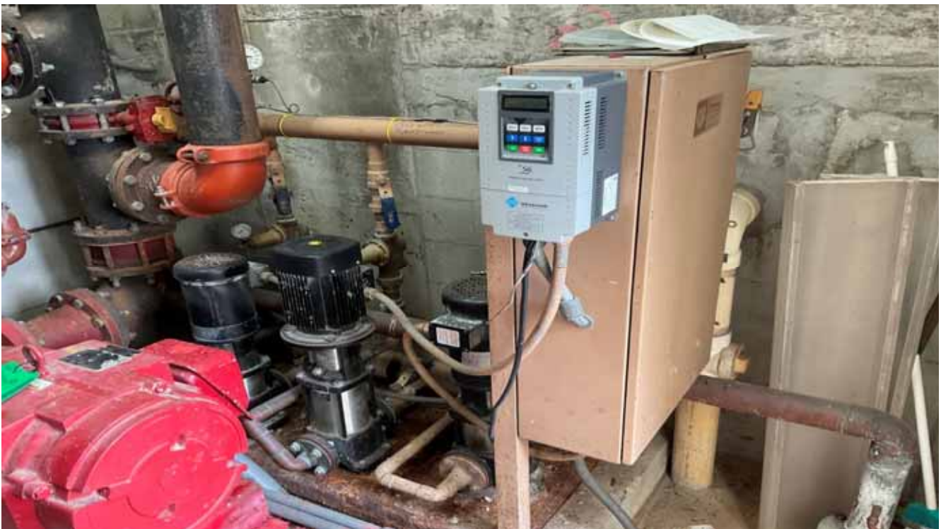
Building D Domestic Water Pump System
