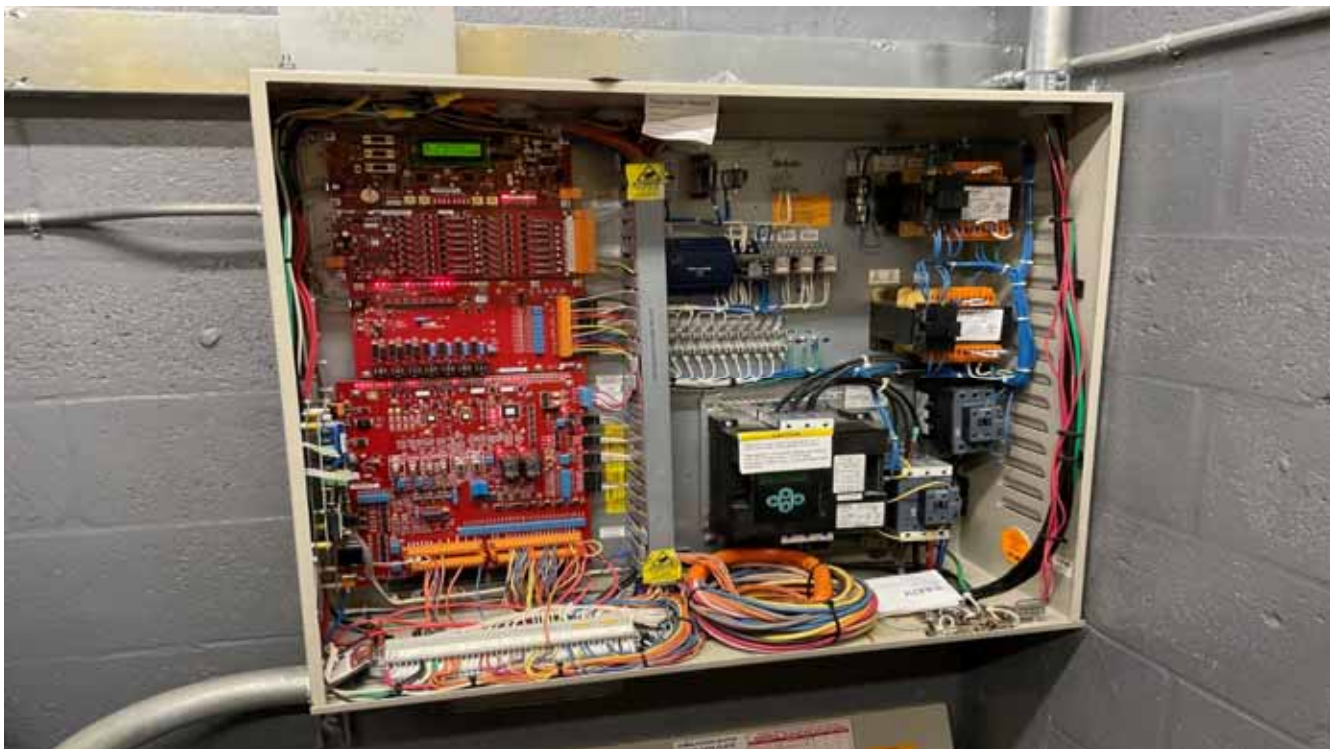
Building E Elevator Equipment
