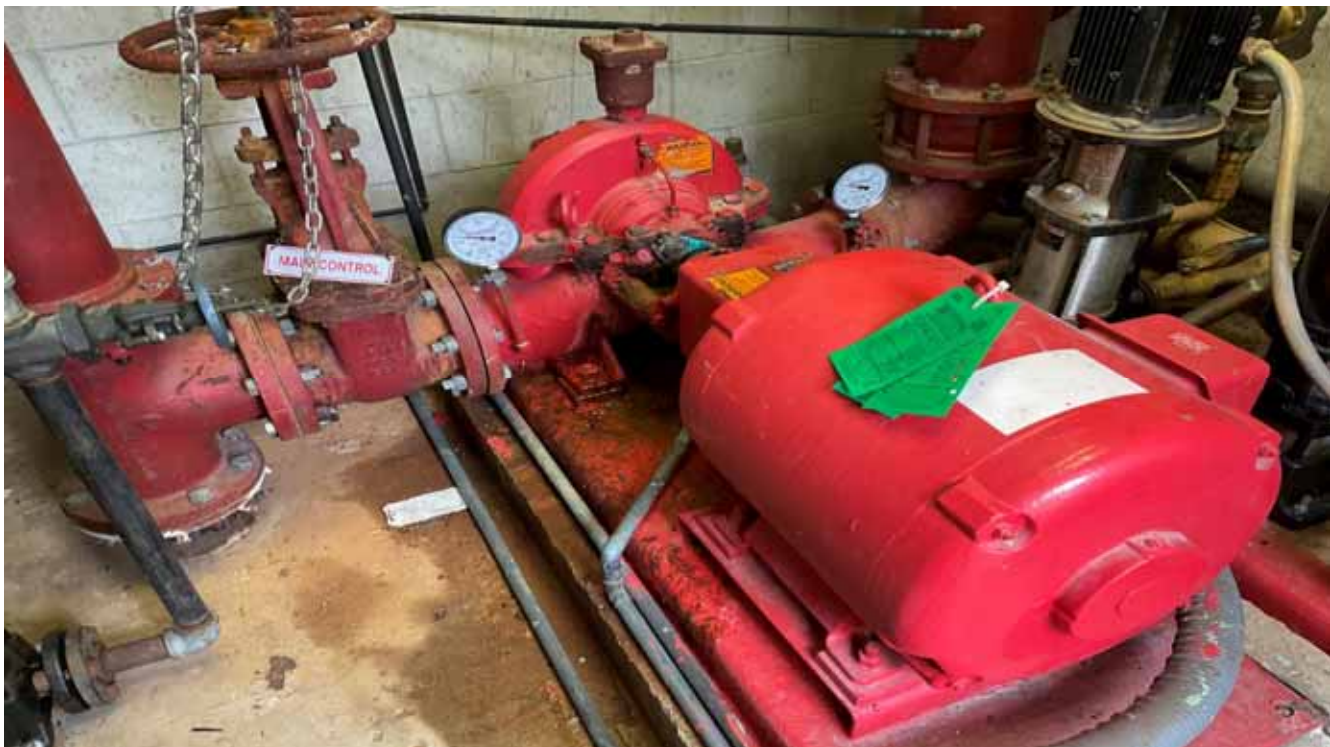
Building F Fire Pump
