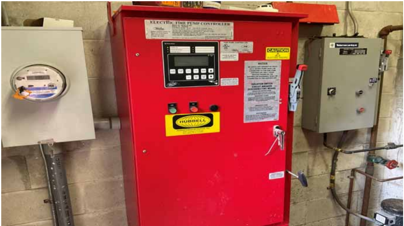
Building H Fire Pump Controller
