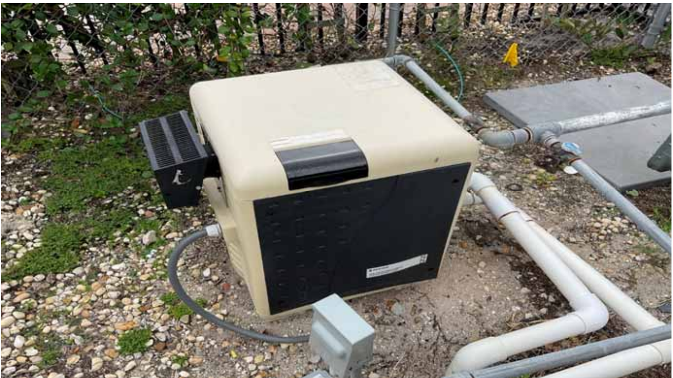
Pool Equipment, Heater
