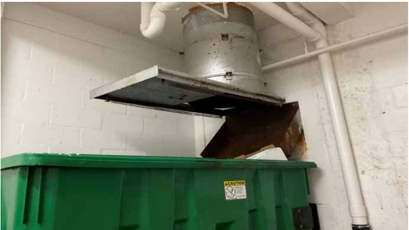
Building F Trash Chute Guillotine
