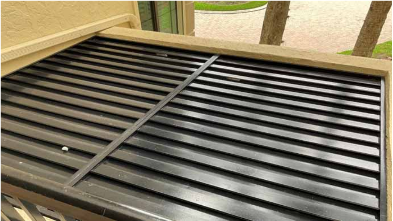
Building H Roof - Pump Room
