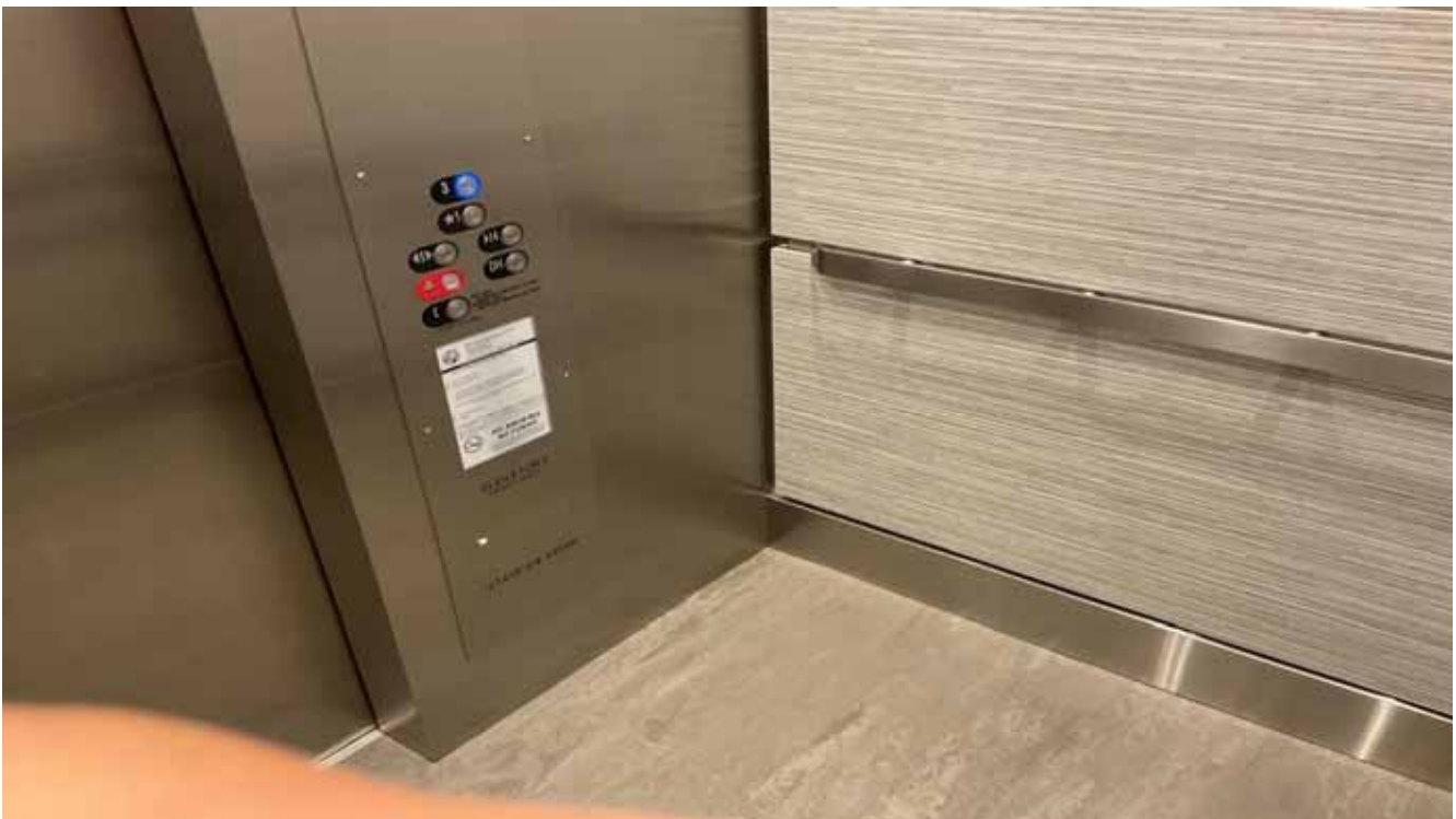
Building E Elevator Cab Interior
