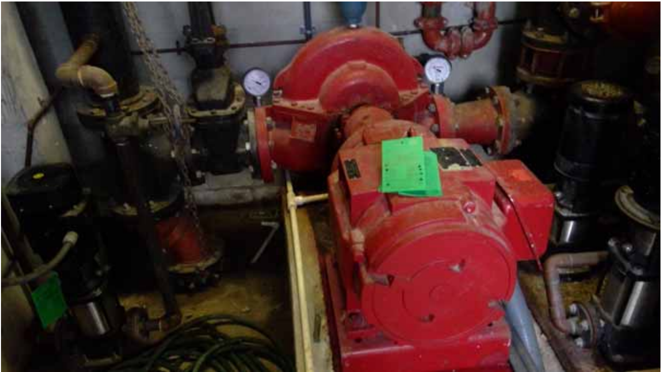
Building D Fire Pump
