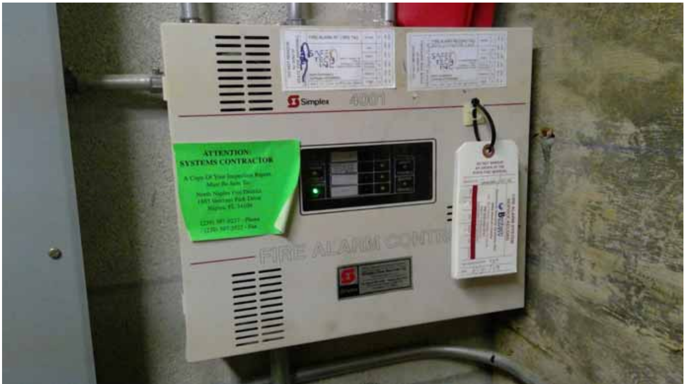
Building E Fire Alarm Control Panel
