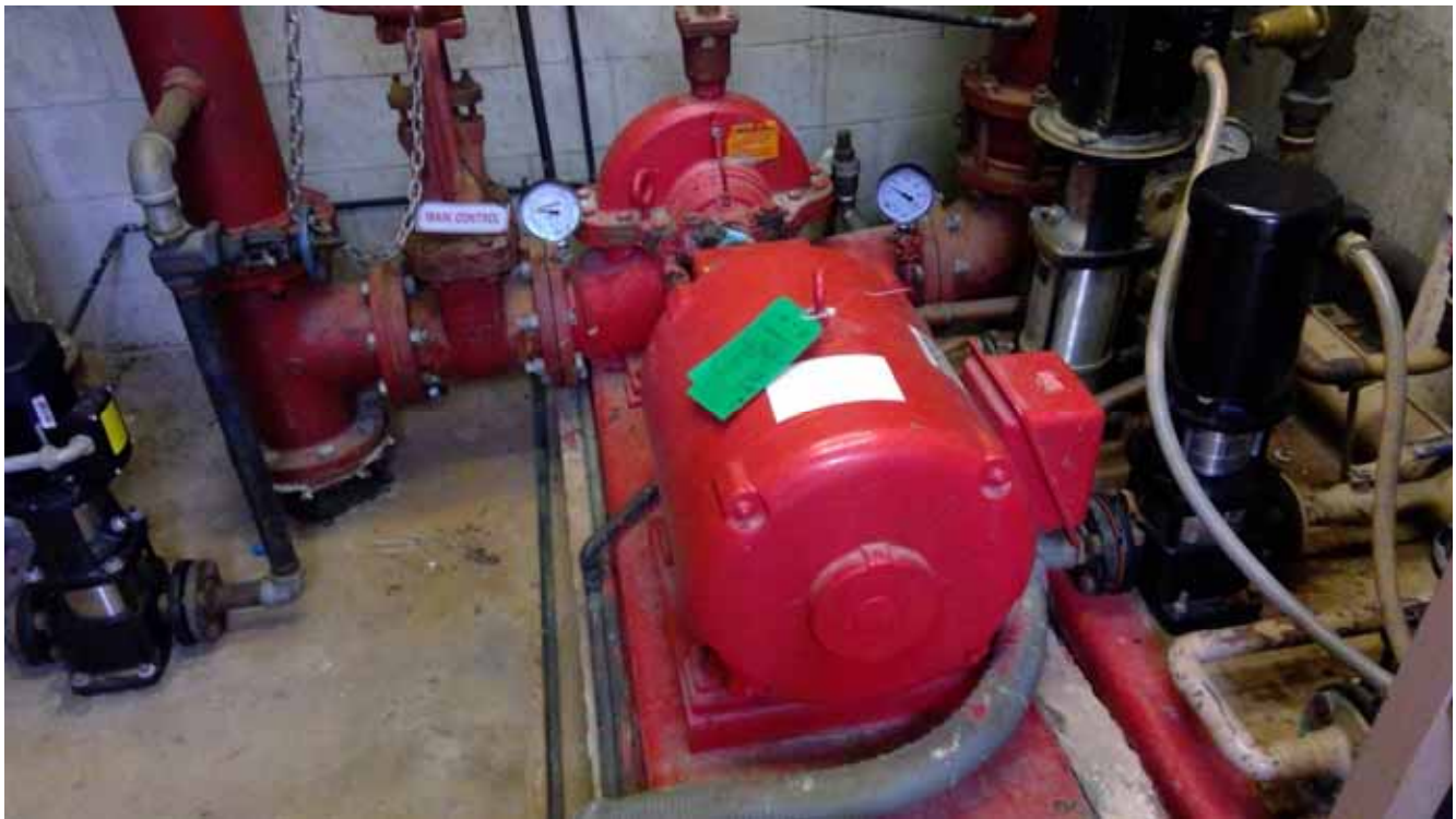
Building F Fire Pump
