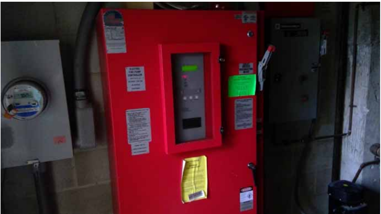
Building D Fire Pump Controller
