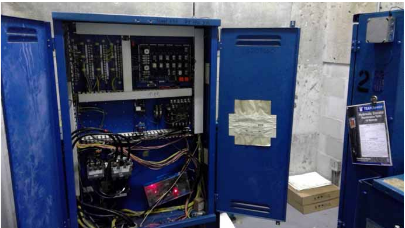
Building D Elevator Equipment
