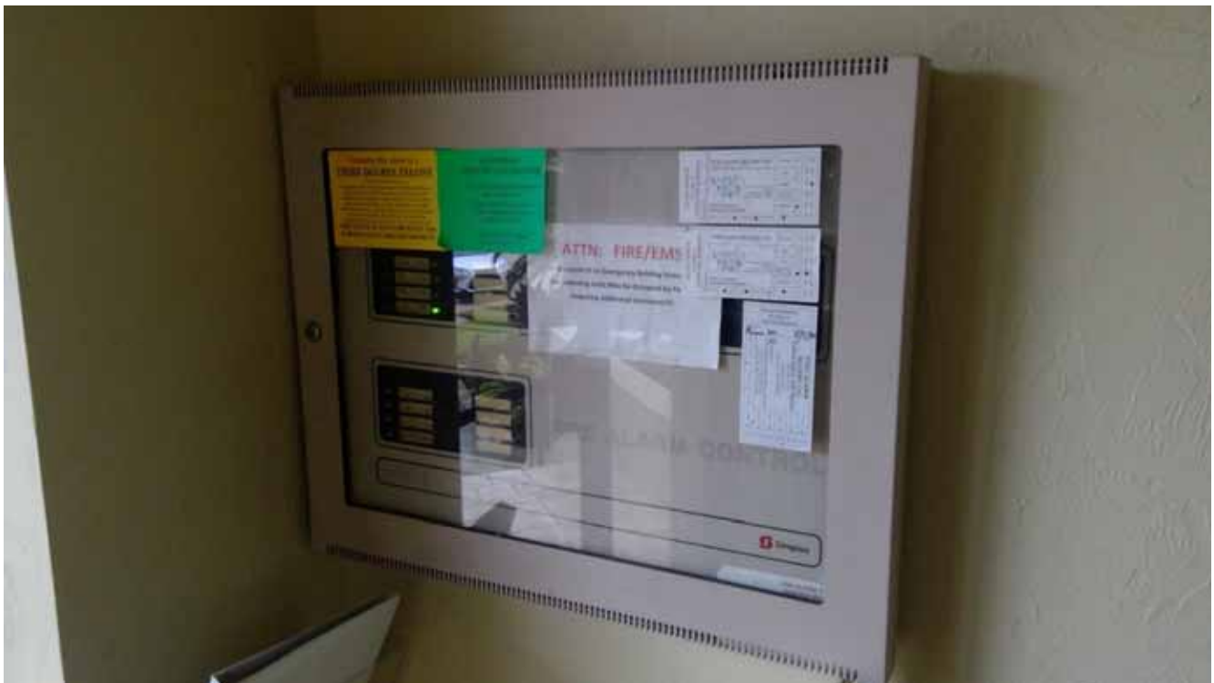
Building F Fire Alarm Control Panel
