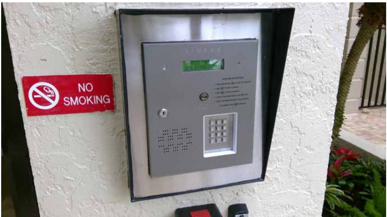
Building F Enterphone
