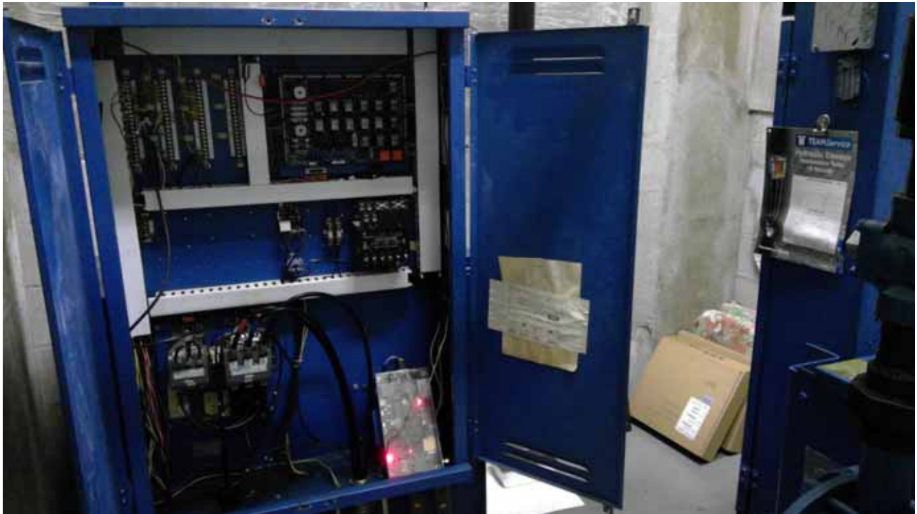
Building H Elevator Equipment
