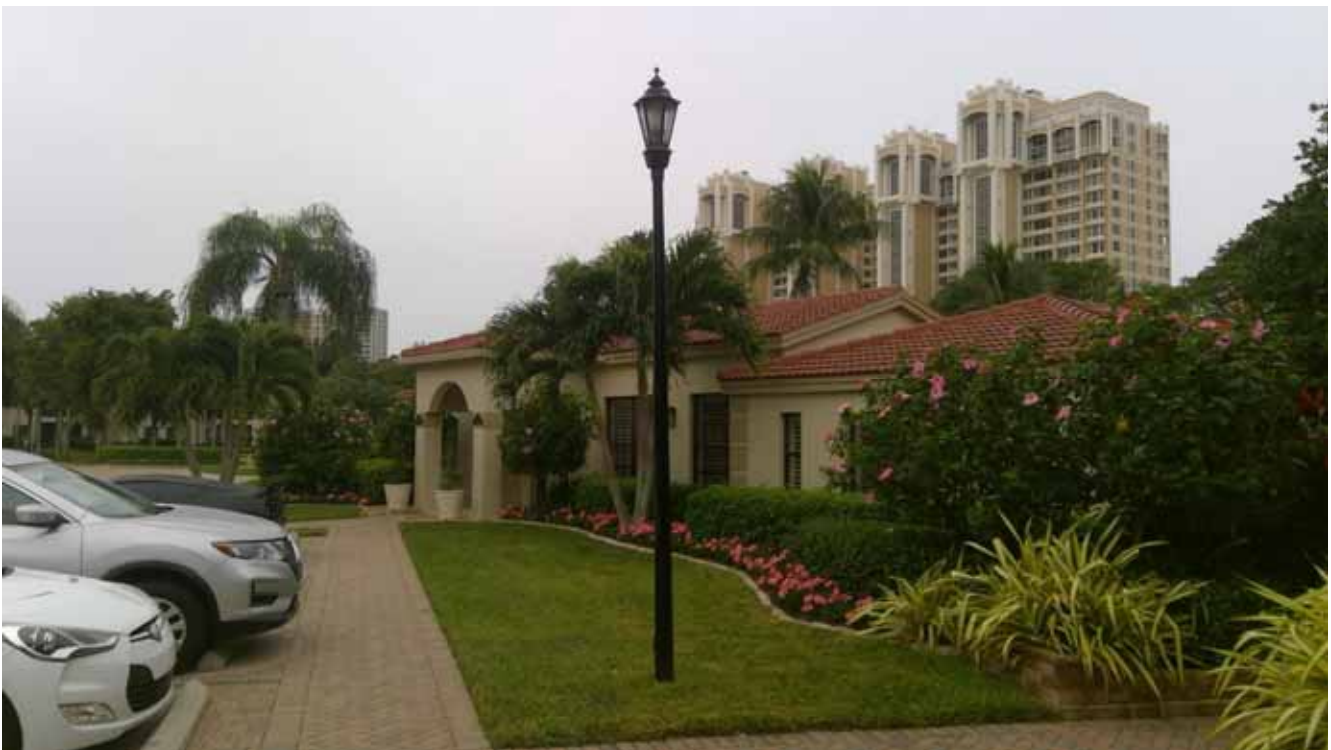
Light Pole & Fixture - Parking Area
