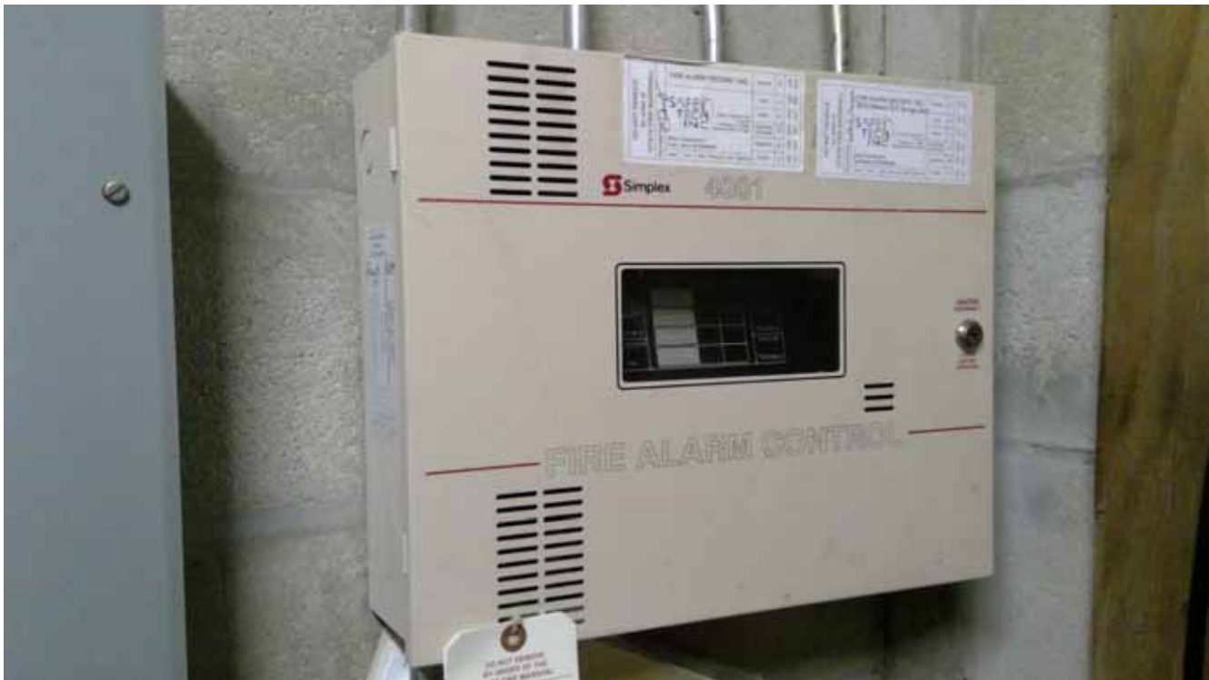
Building C Fire Alarm Control Panel
