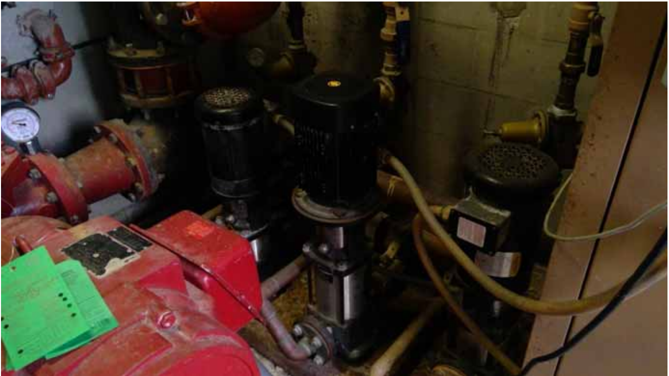
Building D Domestic Water Pump System
