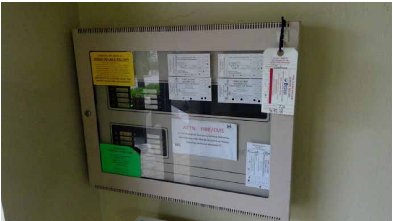
Building H Fire Alarm Control Panel
