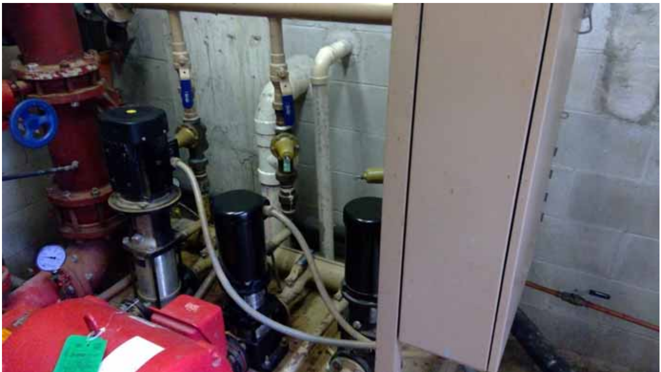
Building F Domestic Water Pump System
