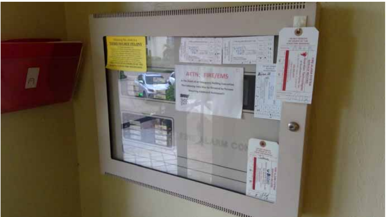
Building D Fire Alarm Control Panel
