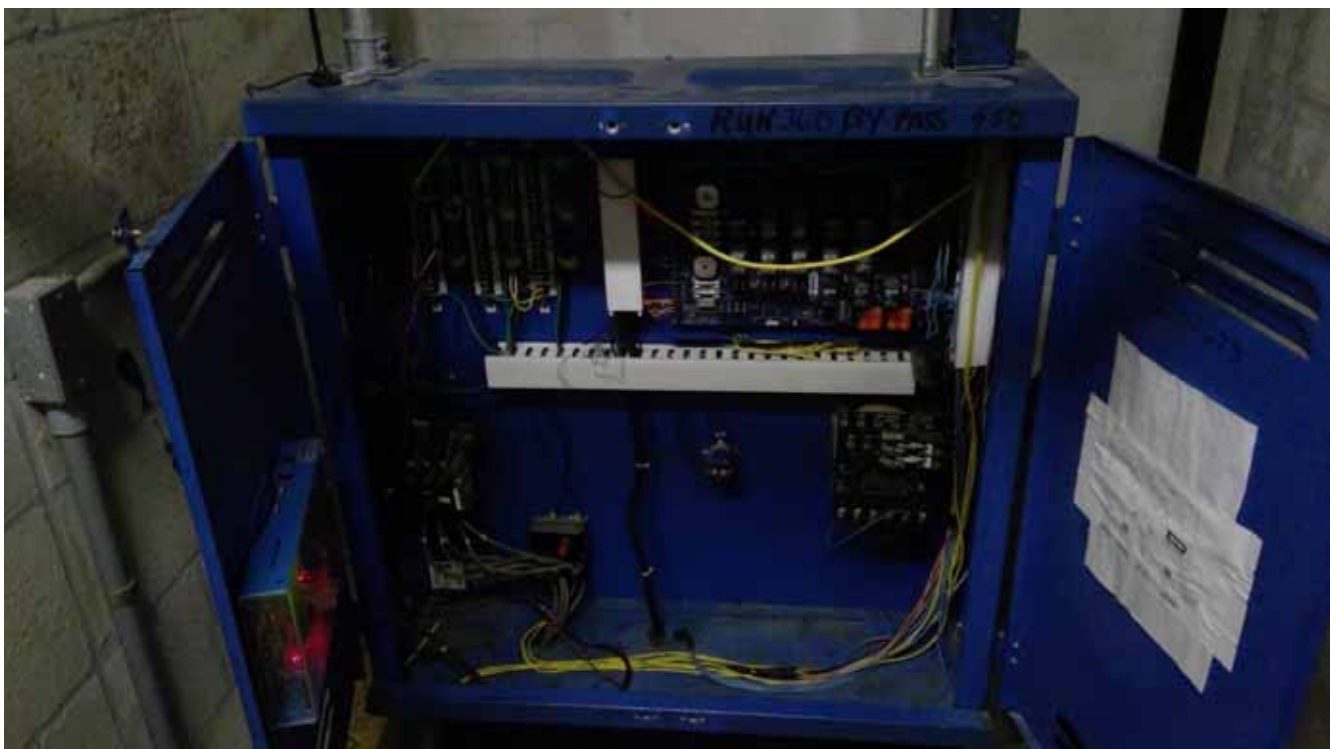
Building C Elevator Equipment
