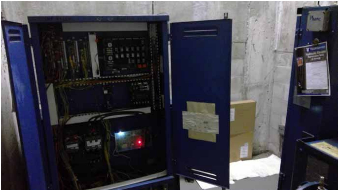
Building F Elevator Equipment
