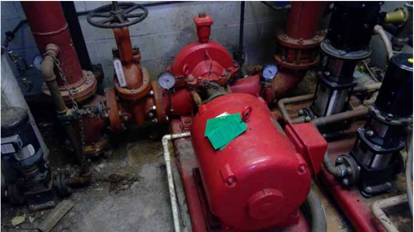
Building H Fire Pump
