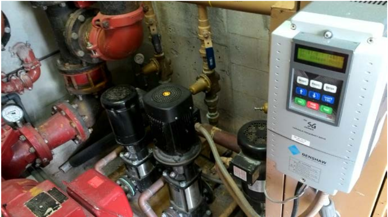
Building D Domestic Water Pump System
