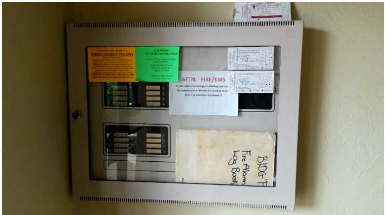
Building F Fire Alarm Control Panel
