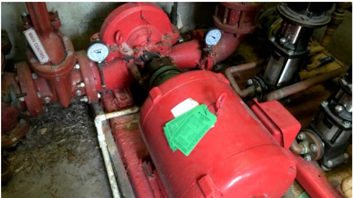
Building H Fire Pump
