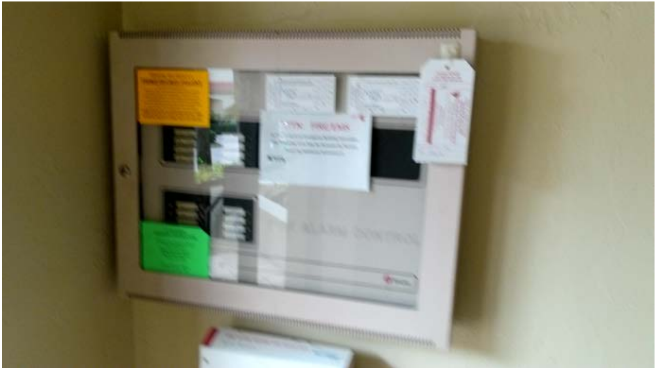
Building H Fire Alarm Control Panel
