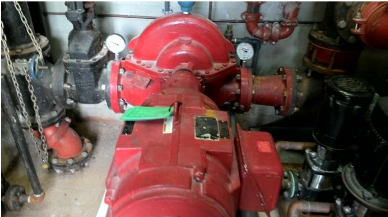
Building D Fire Pump
