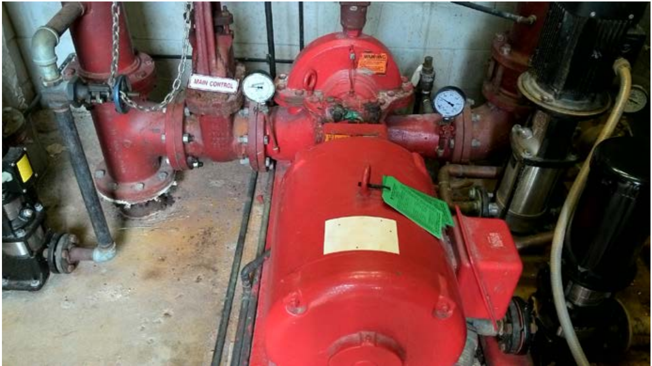
Building F Fire Pump
