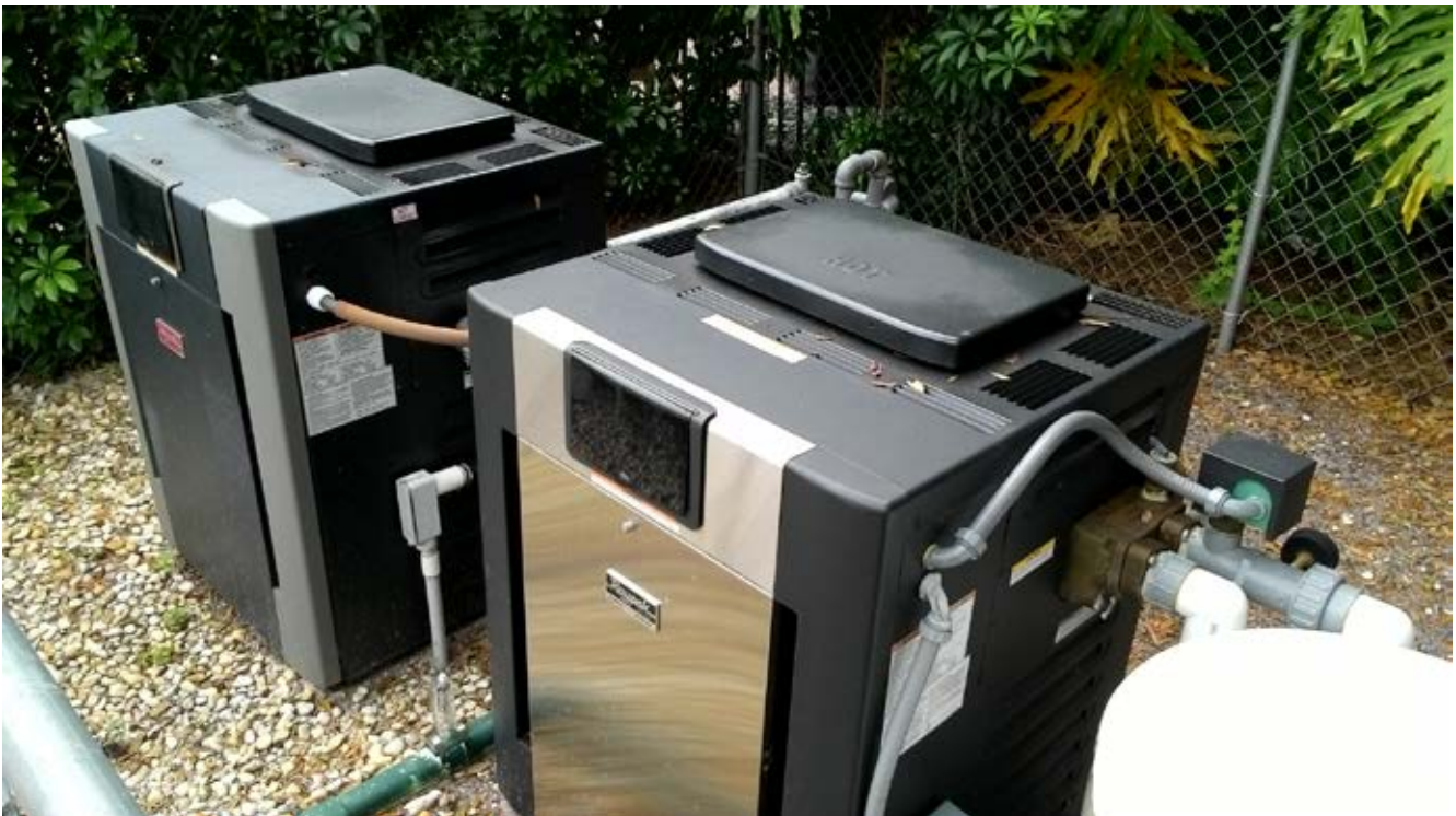
Swimming Pool and Spa Equipment, Heaters
