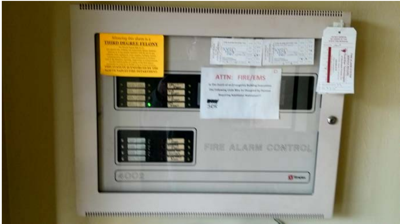
Building D Fire Alarm Control Panel
