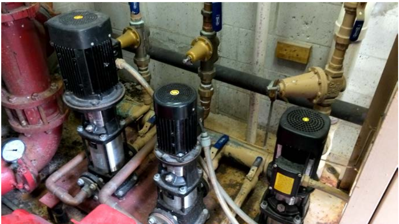
Building H Domestic Water Pump System
