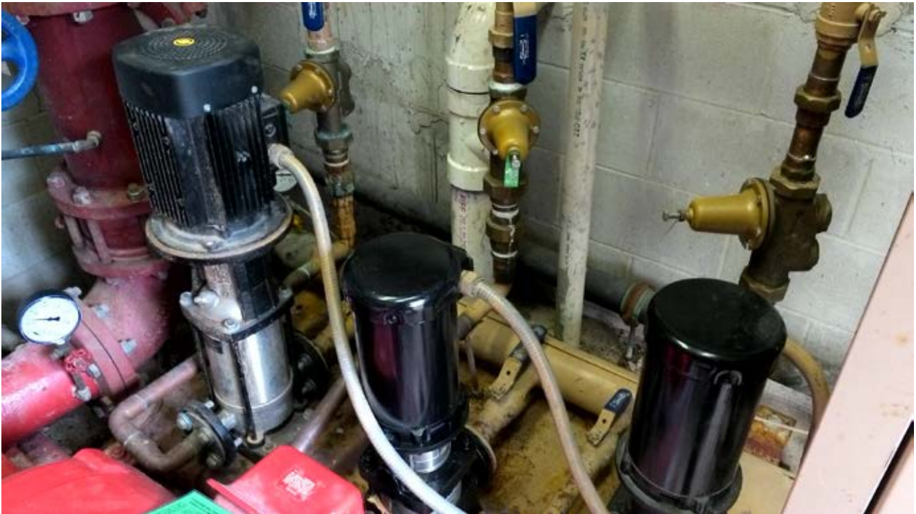
Building F Domestic Water Pump System
