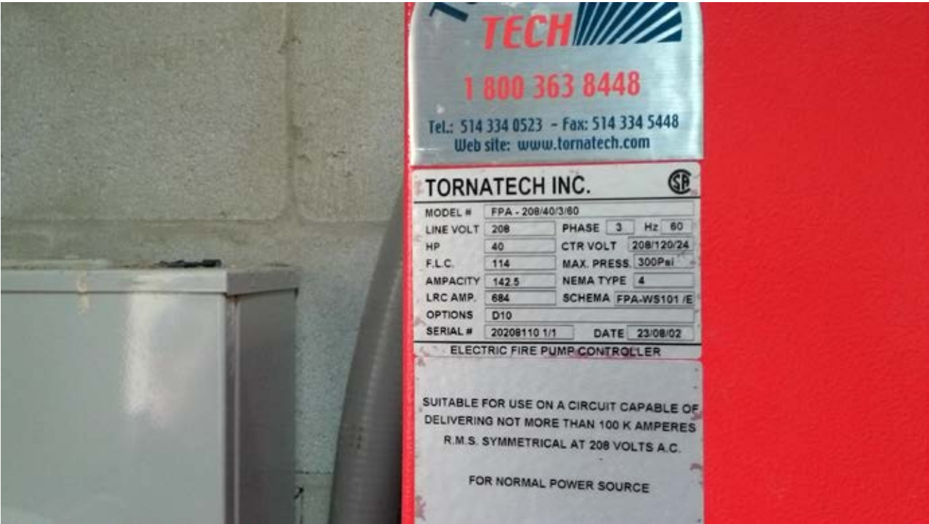
Building D Fire Pump Controller
