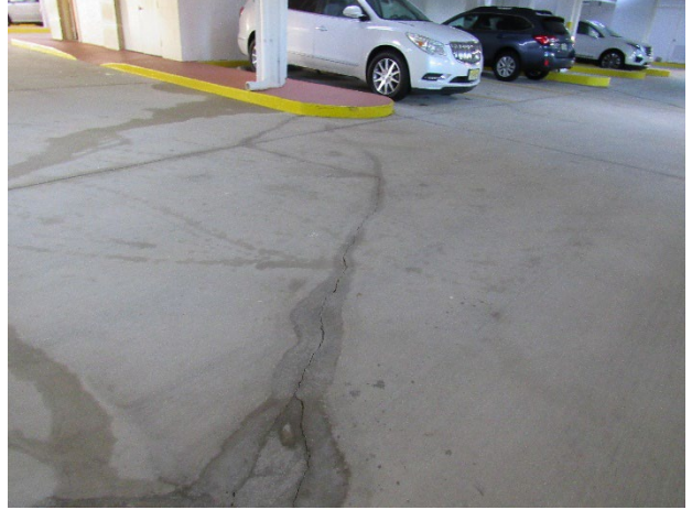
Garage slab crack, Building F
