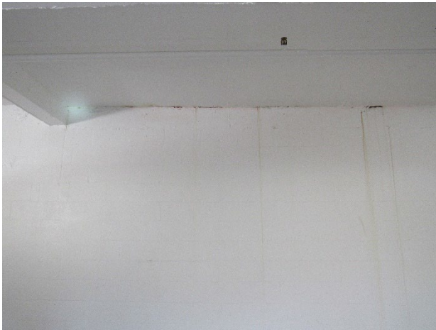
Active water intrusion, building F garage
