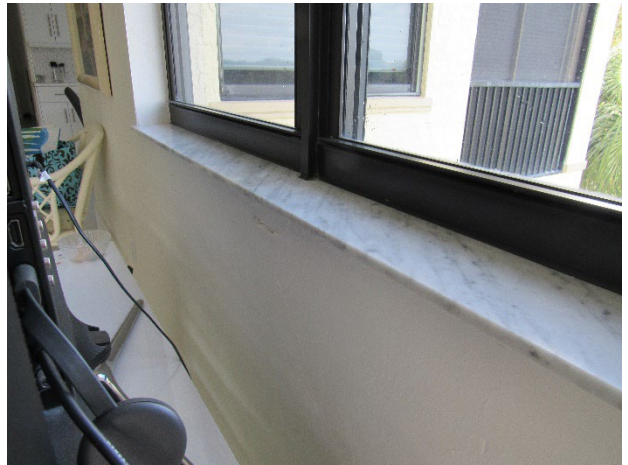
Water intrusion signs, Unit F303
