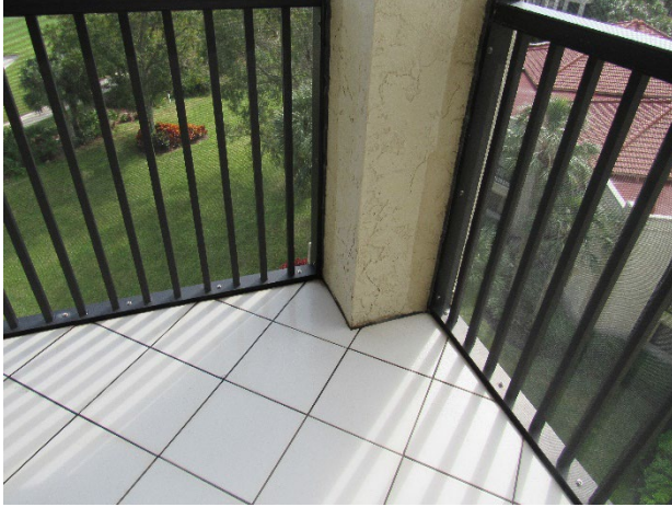
Typical stucco spall at column, Unit F502
