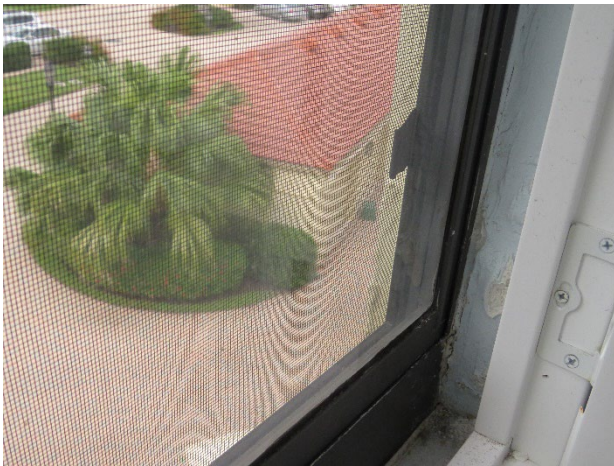
Water intrusion, Unit E301
