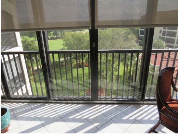
Enclosed balcony, delaminated tile, Units E501
