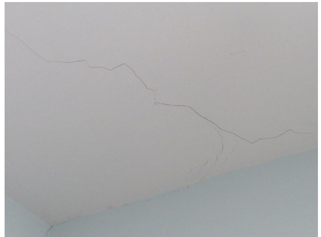
Ceiling crack, Unit E301
