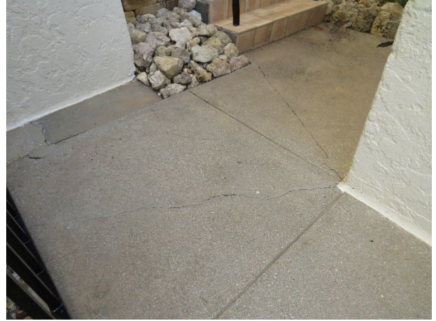
Settlement, slab cracking, building E
