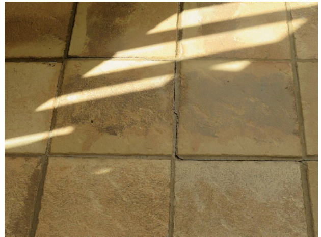
Delaminated tile in E corridor, 2 nd floor
