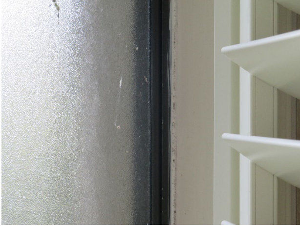
Apparent mold at window sealant, Unit C105
