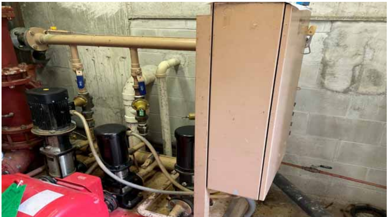
Building F Domestic Water Pump System
