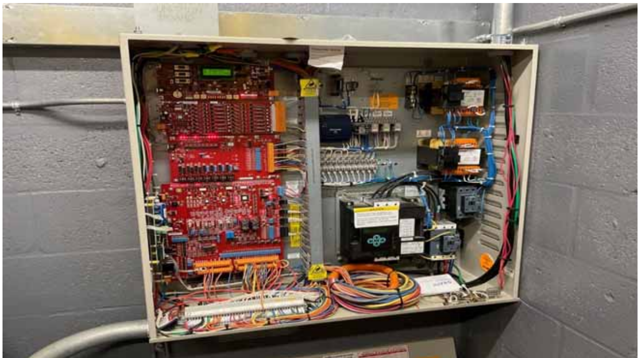
Building E Elevator Equipment
