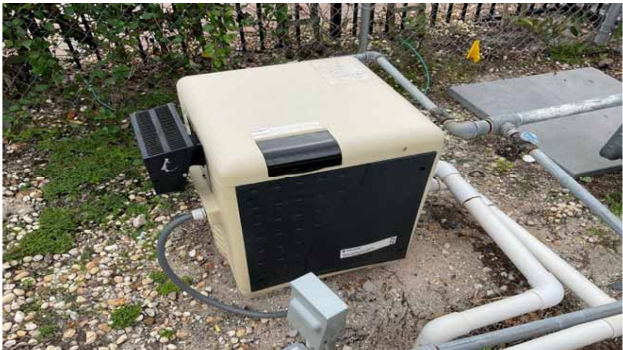
Pool Equipment, Heater
