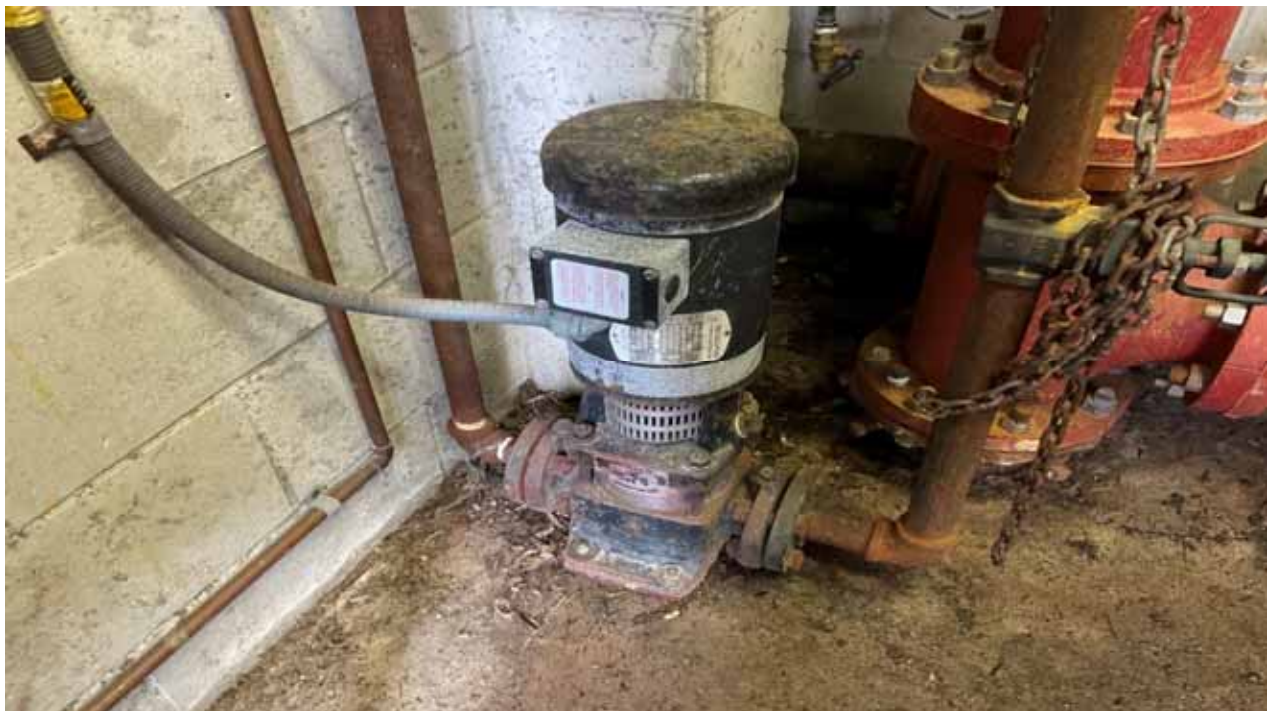
Building H Fire Jockey Pump
