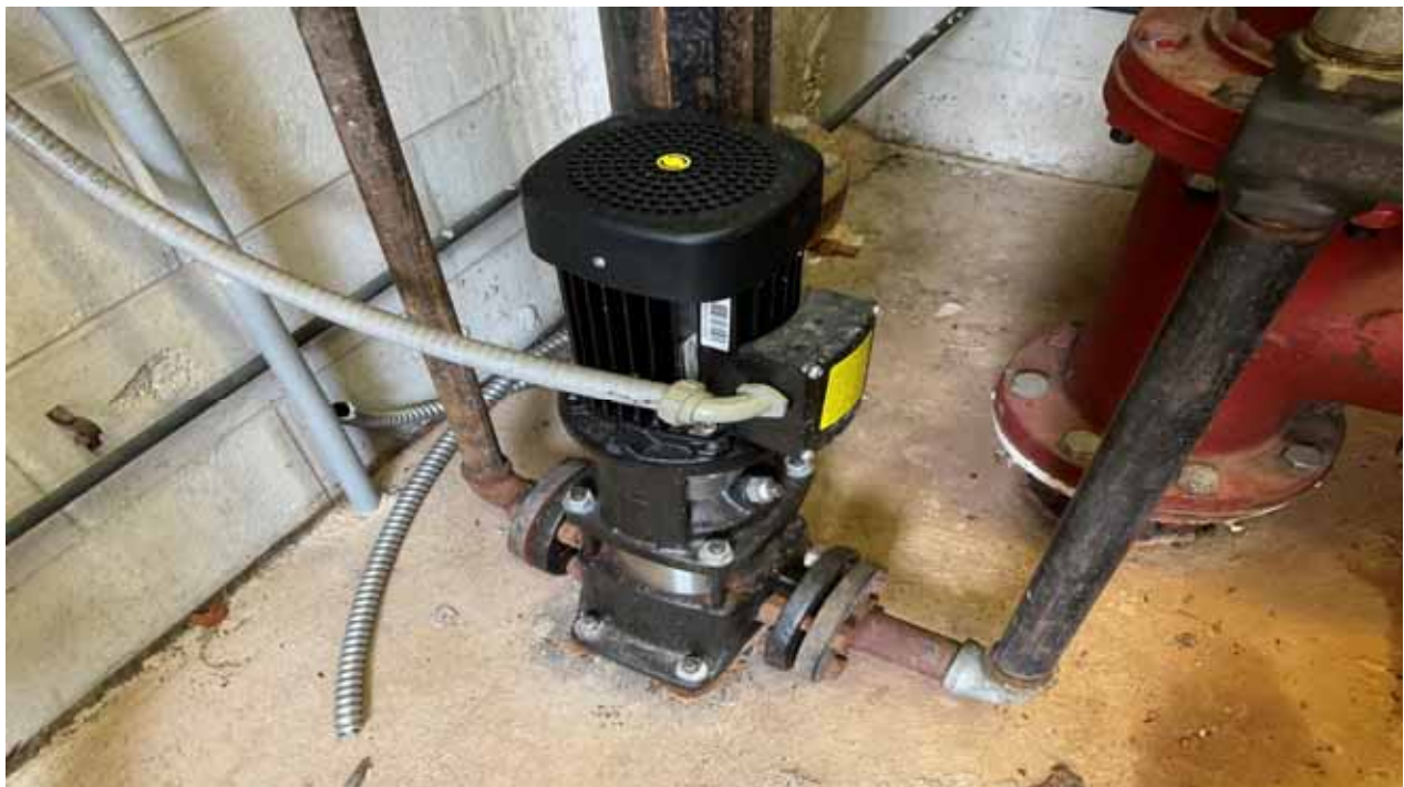
Building F Fire Jockey Pump
