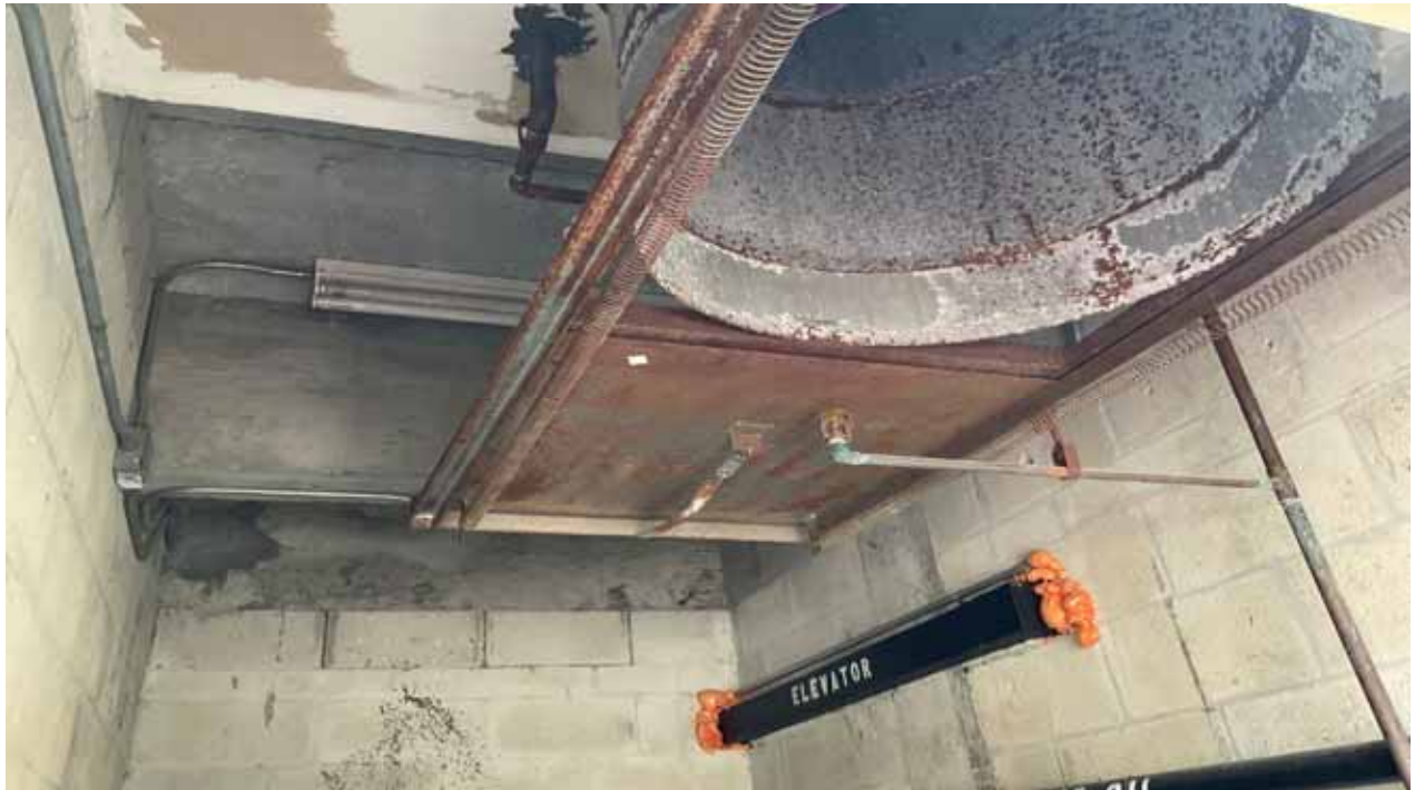
Building E Trash Chute Guillotine
