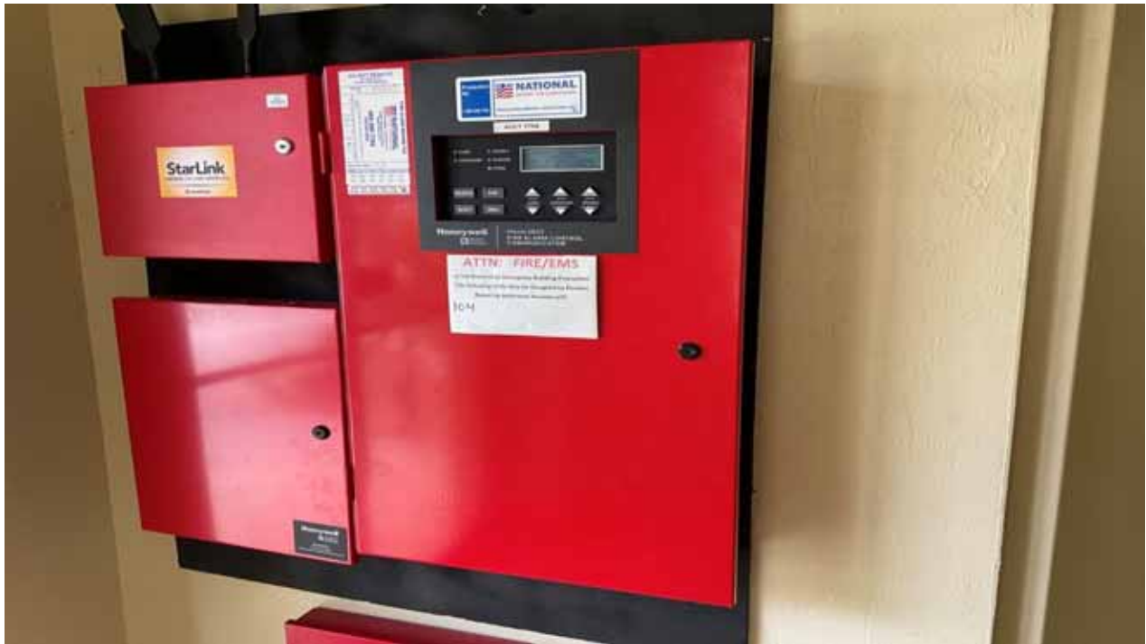
Building D Fire Alarm Panel
