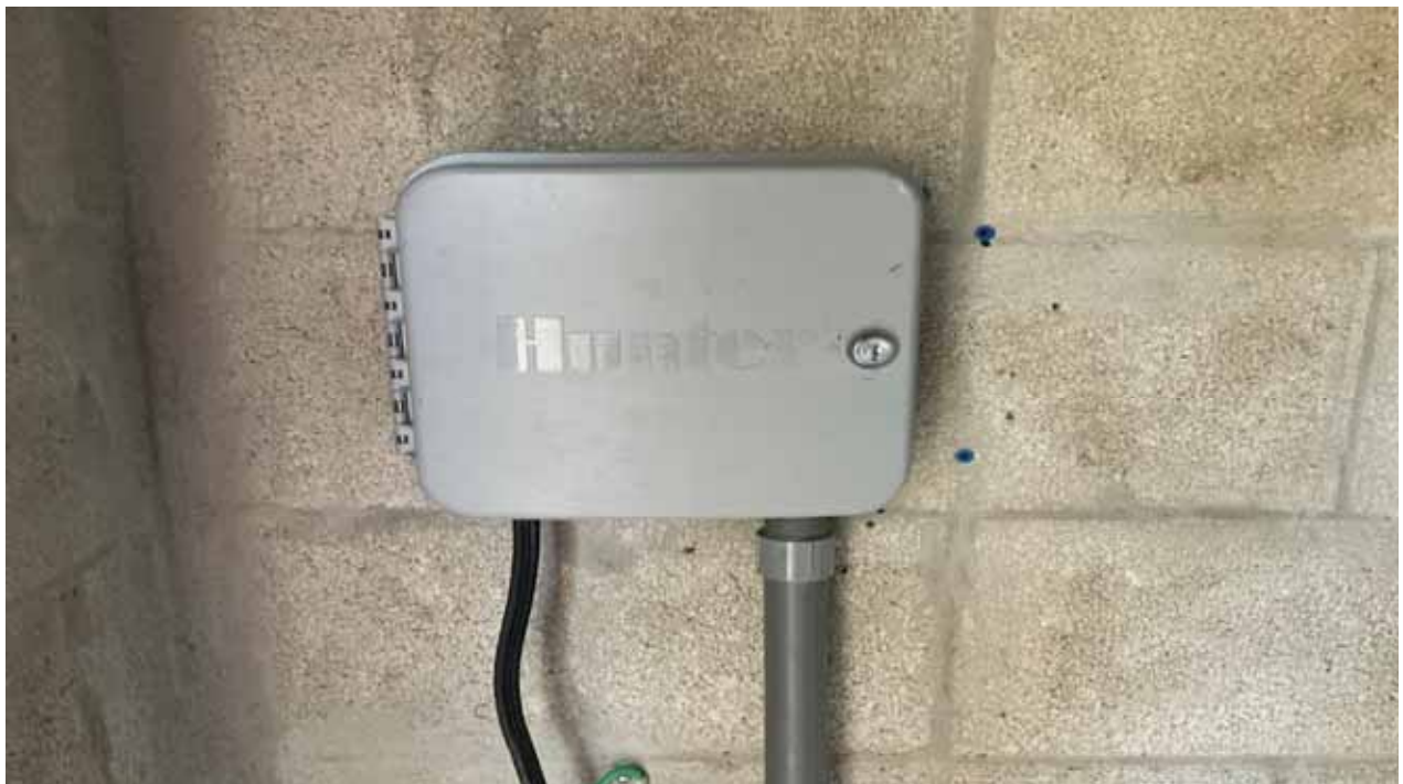
Irrigation Control Station (1 of 6)
