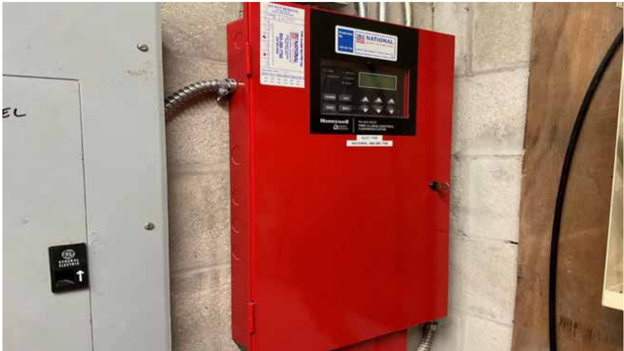
Building C Fire Alarm Panel
