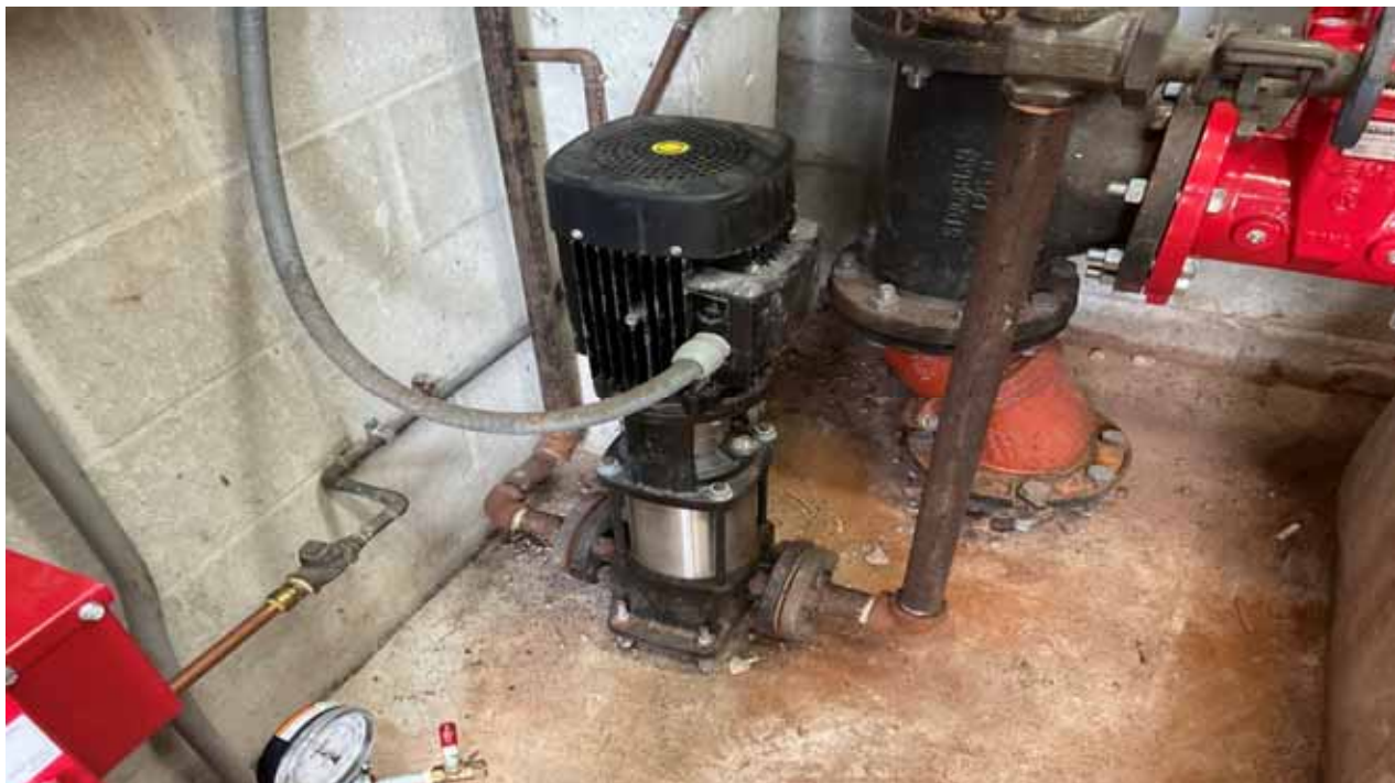
Building D Fire Jockey Pump
