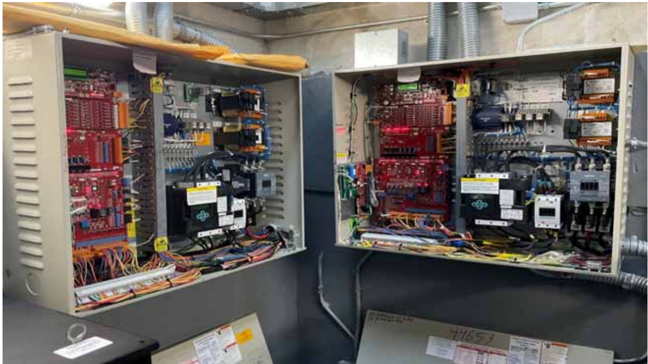
Building H Elevator Equipment
