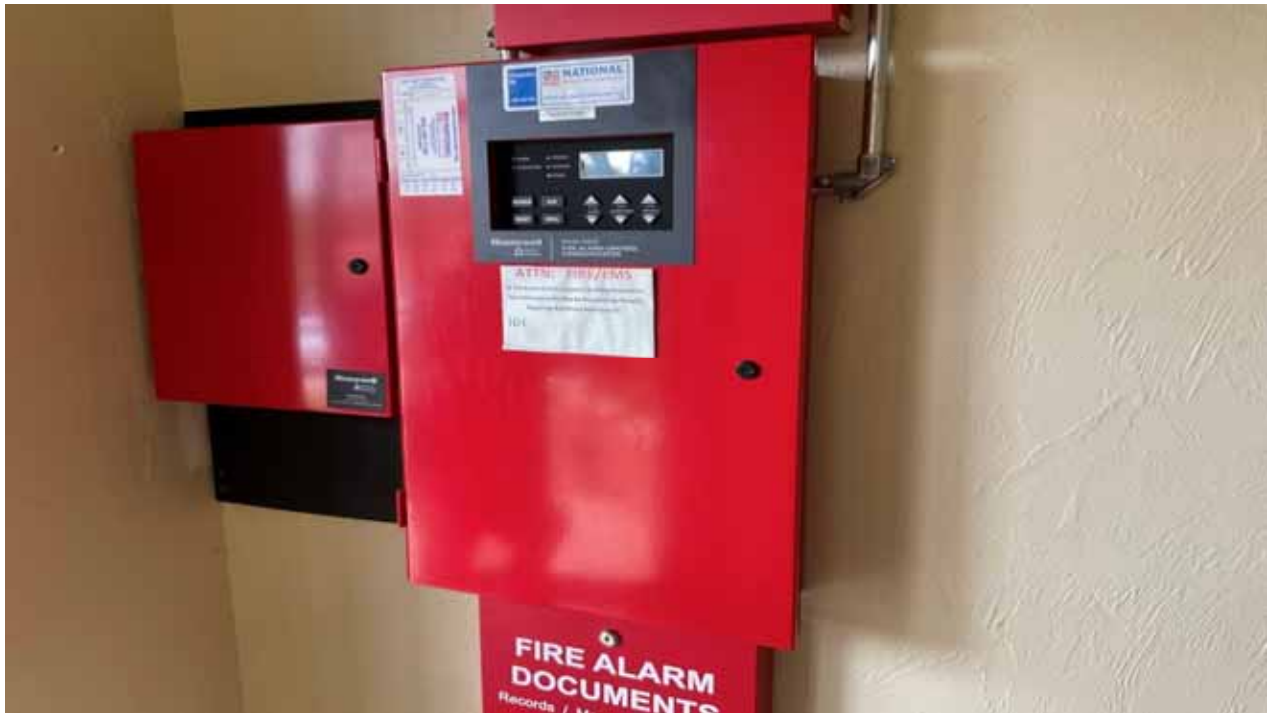
Building F Fire Alarm Panel
