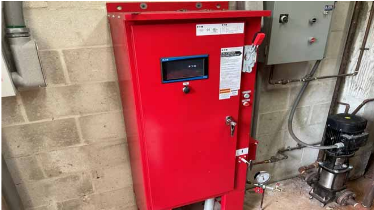
Building D Fire Pump Controller
