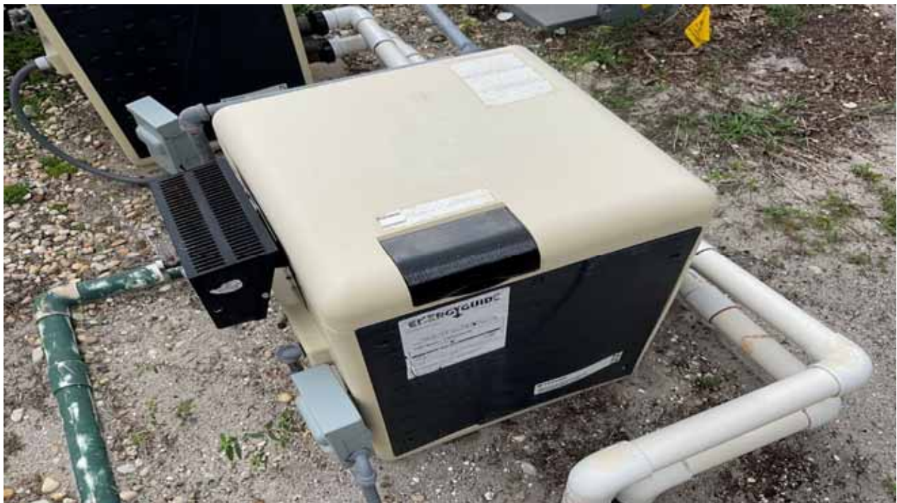
Spa Equipment, Heater
