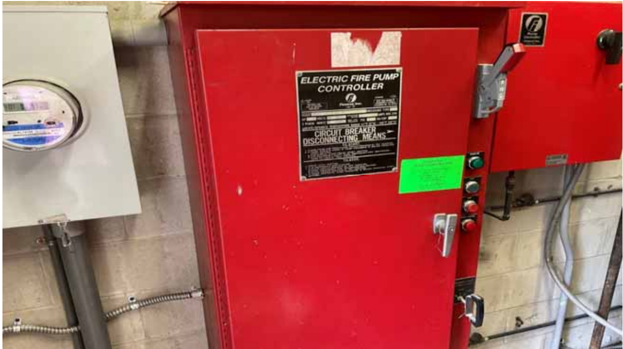
Building F Fire Pump Controller
