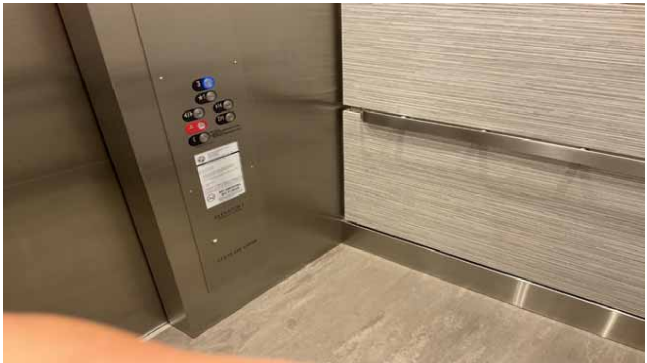
Building E Elevator Cab Interior
