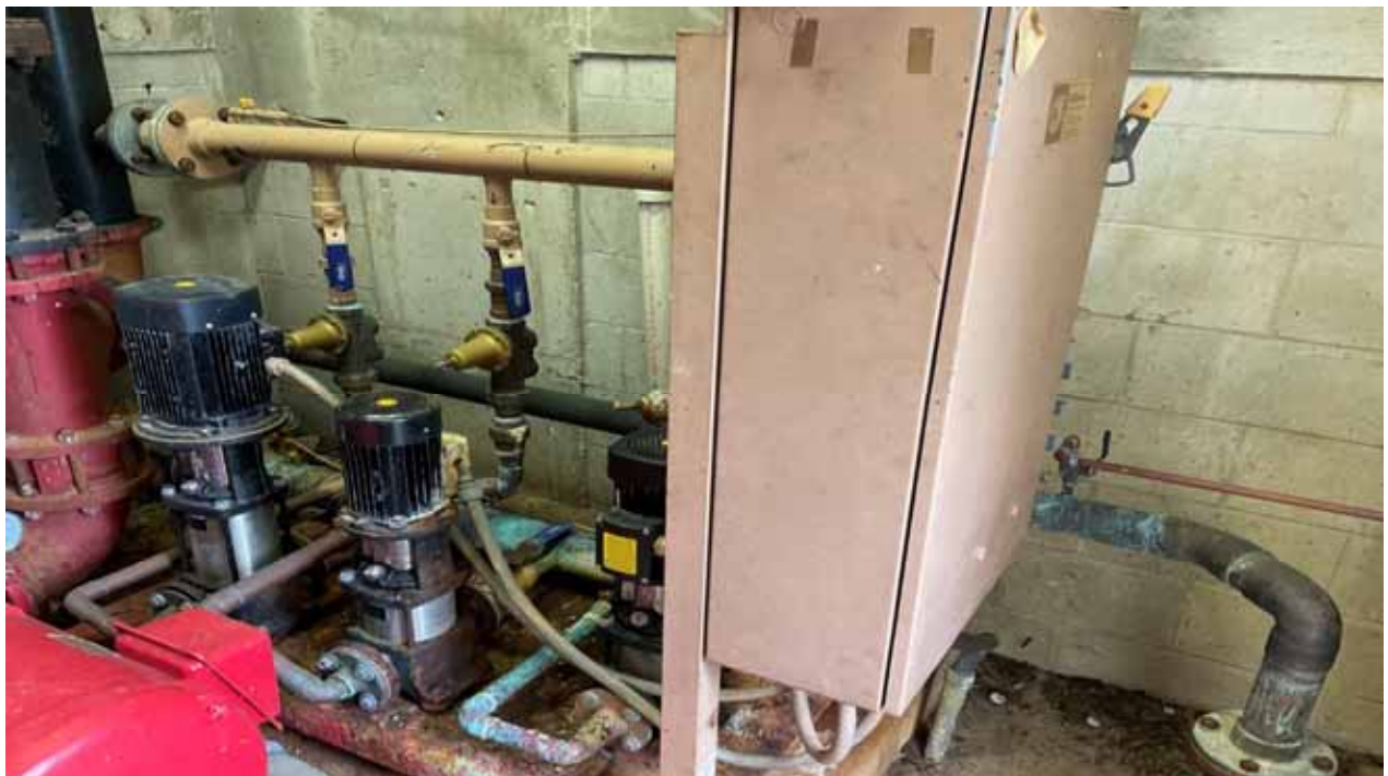
Building H Domestic Water Pump System
