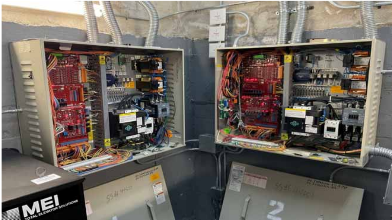
Building F Elevator Equipment
