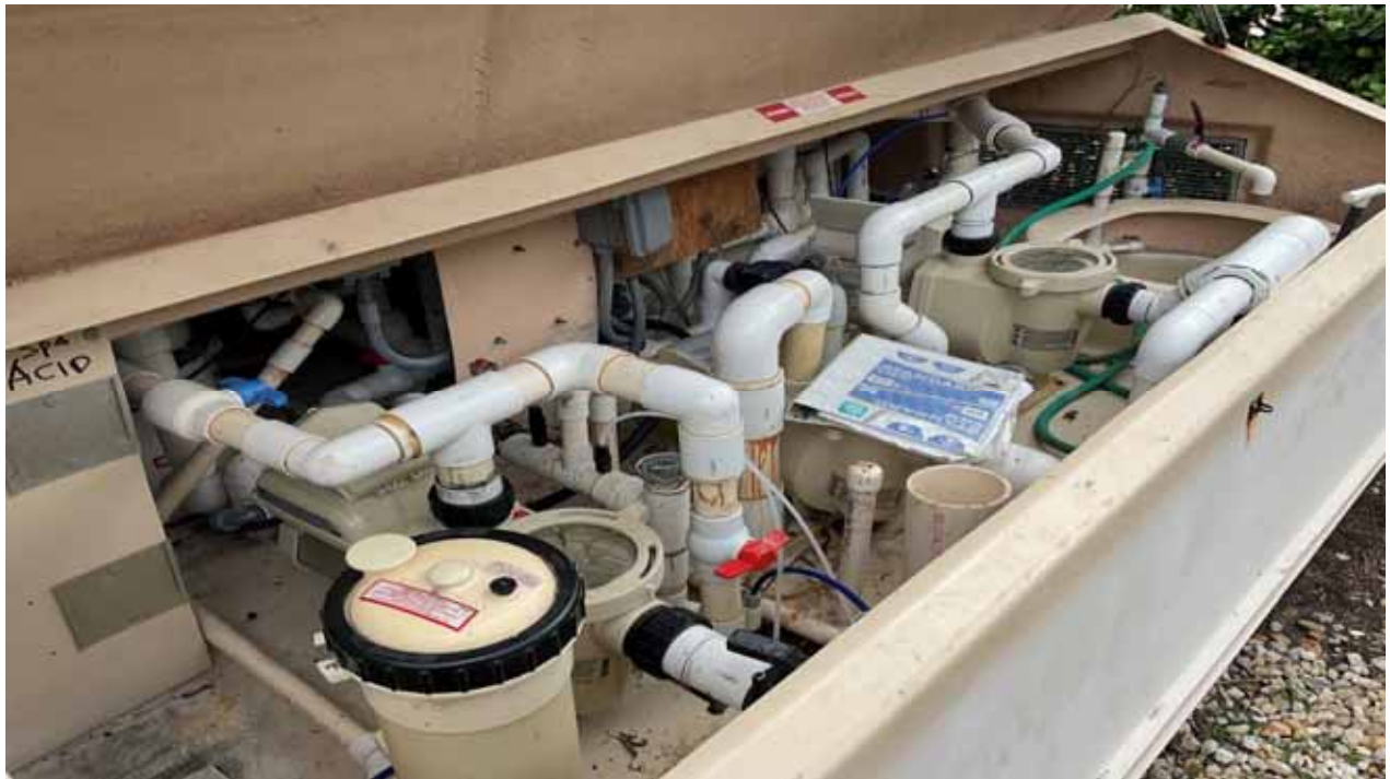
Pool & Spa Equipment
