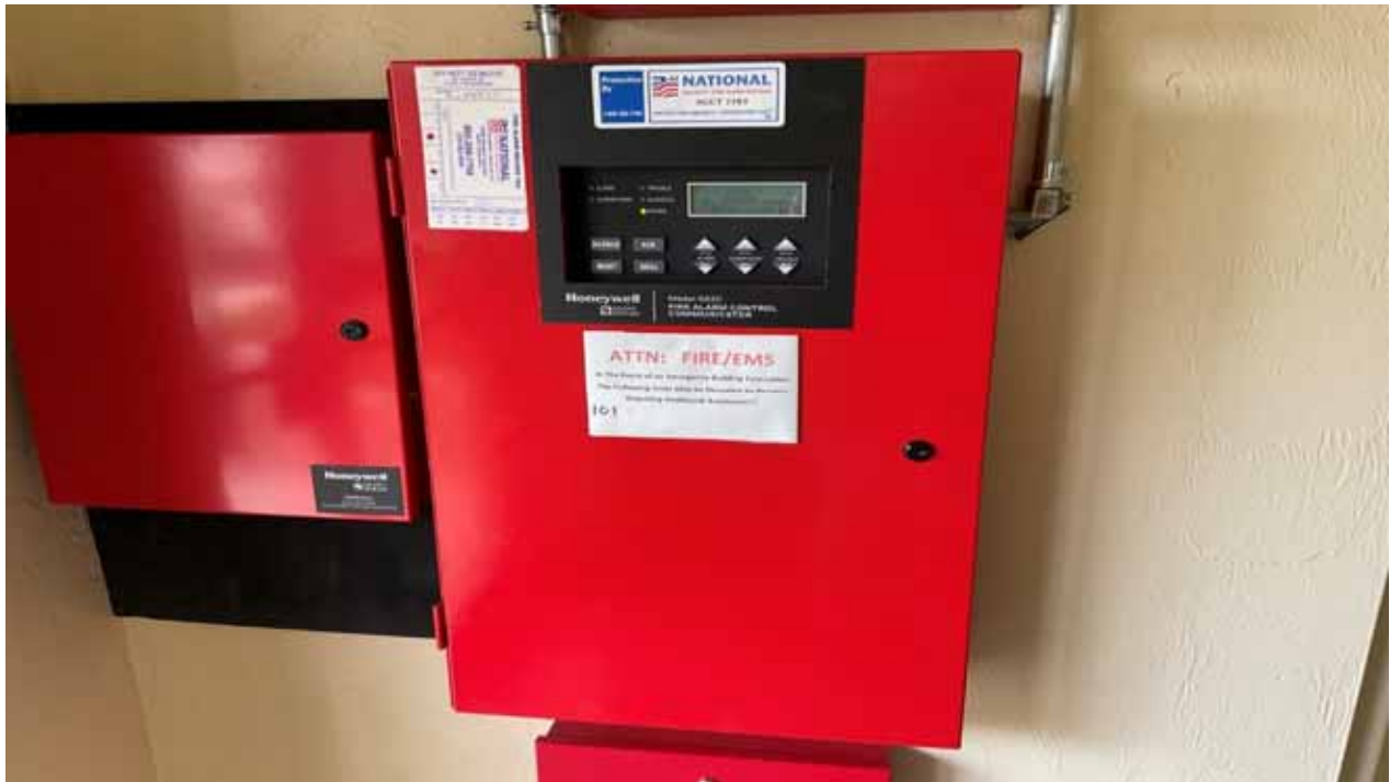
Building H Fire Alarm Panel
