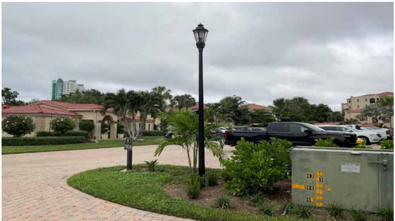
Light Pole & Fixture - Parking Lot
