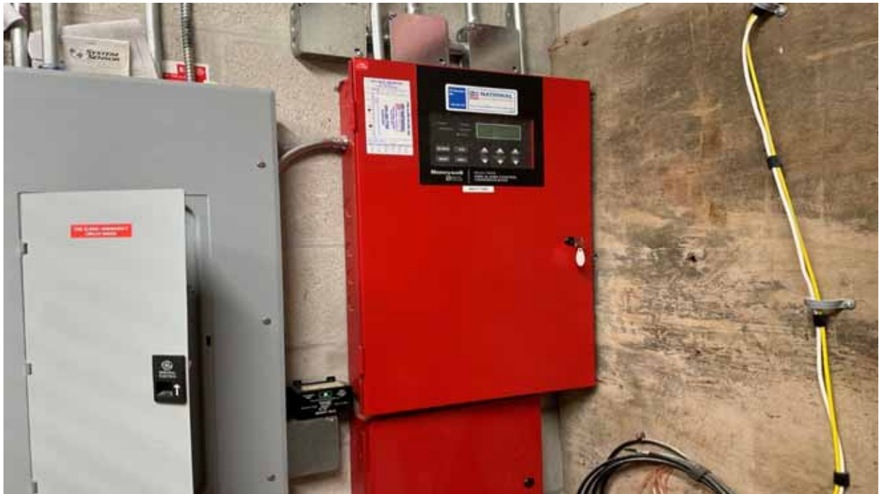
Building E Fire Alarm Panel
