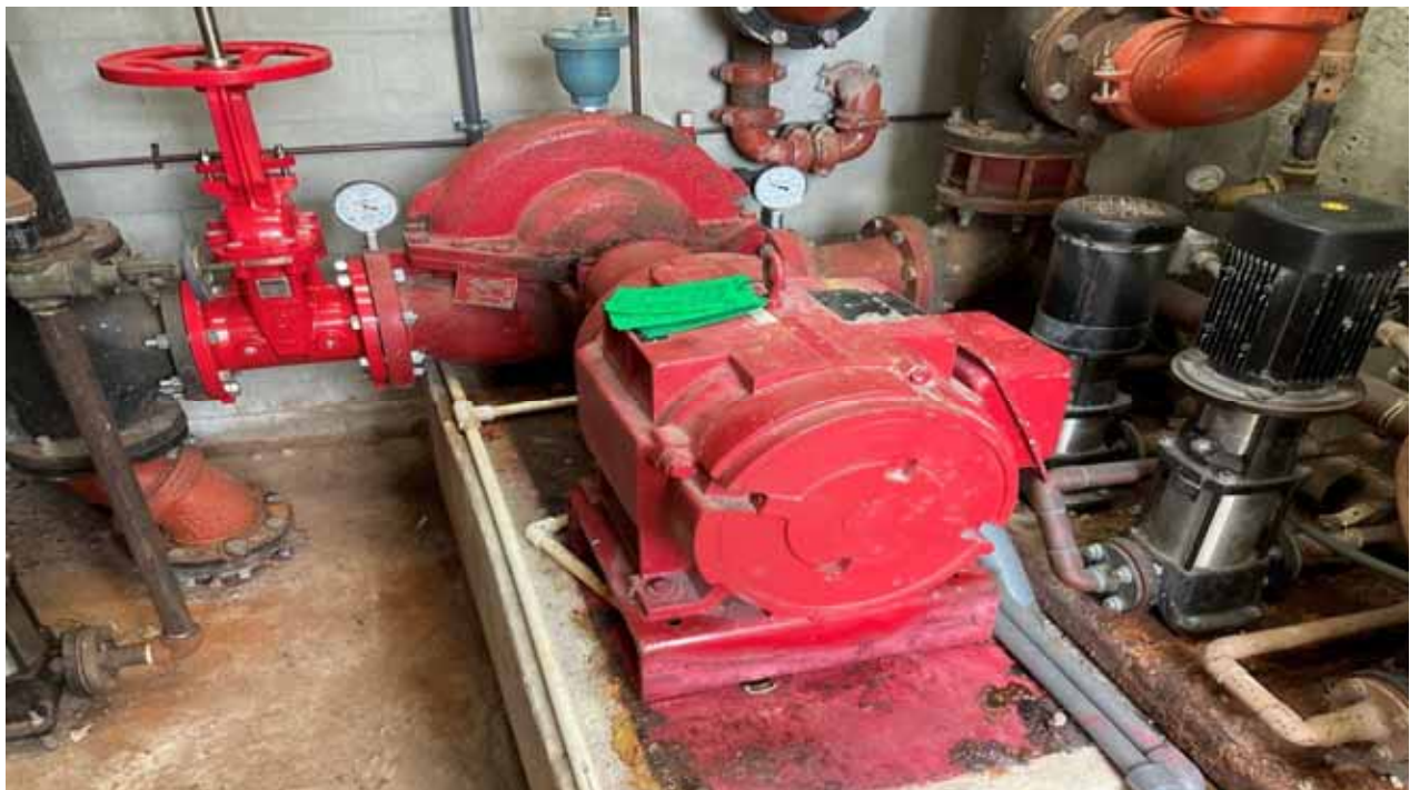
Building D Fire Pump
