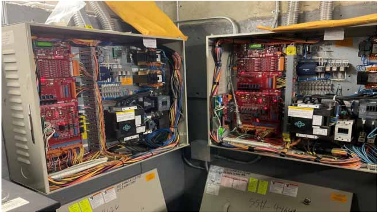
Building D Elevator Equipment
