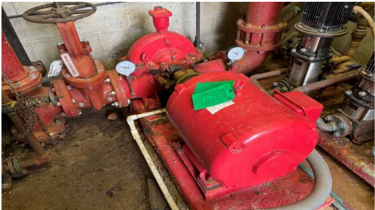
Building H Fire Pump
