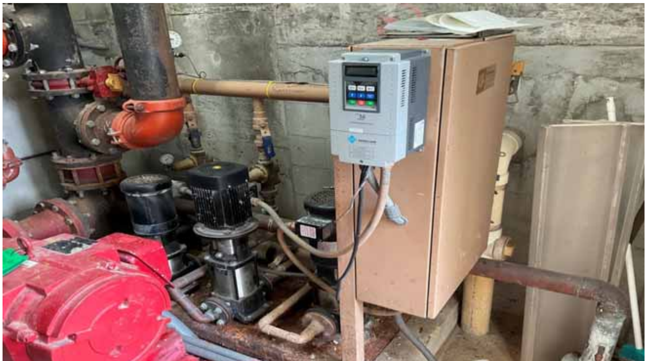
Building D Domestic Water Pump System
