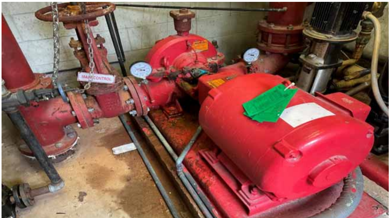
Building F Fire Pump
