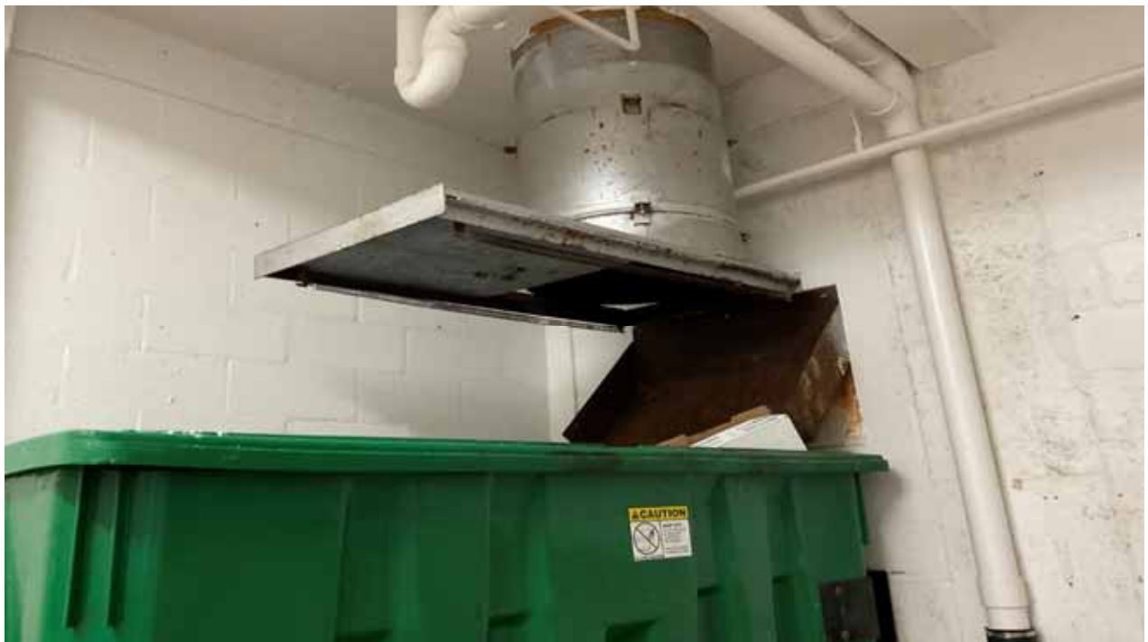
Building F Trash Chute Guillotine
