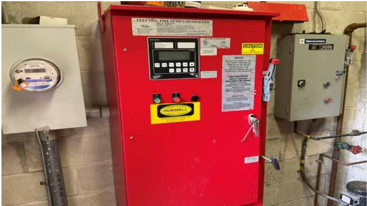
Building H Fire Pump Controller
